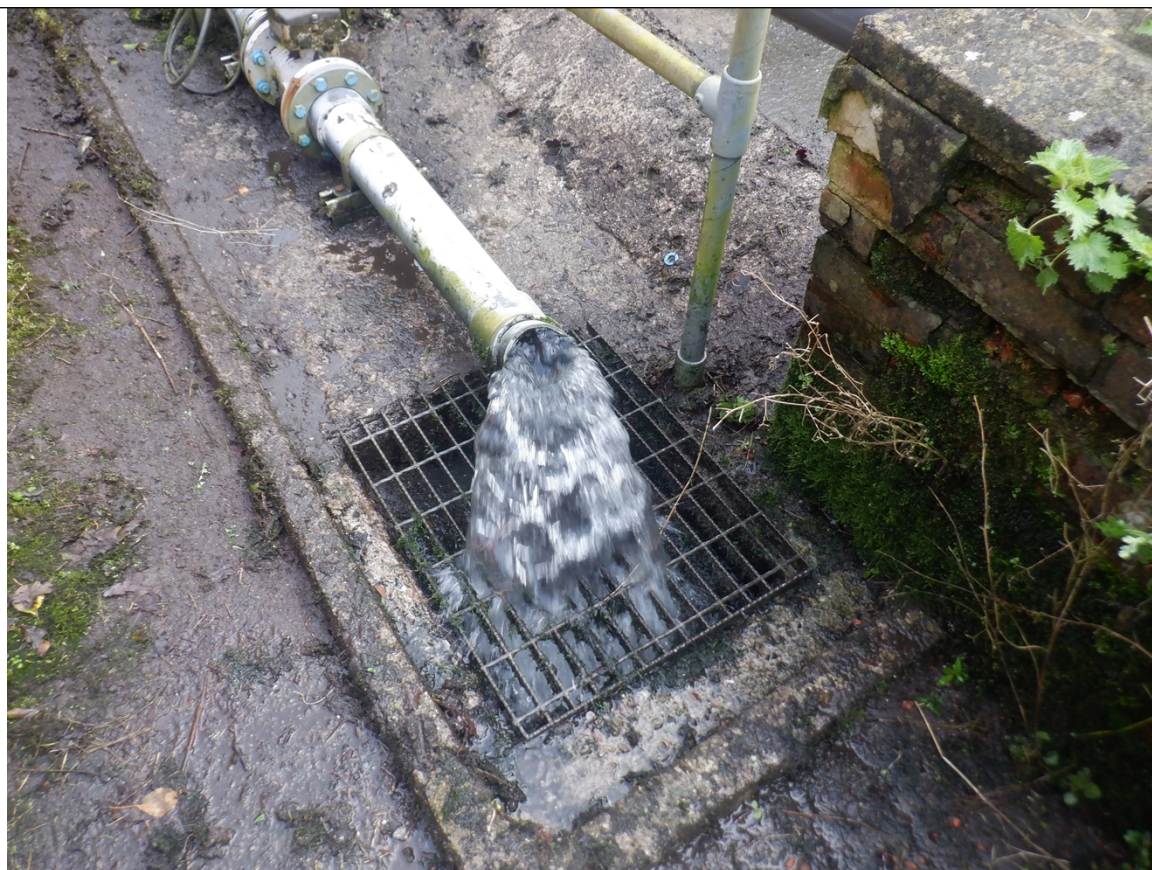
Photo showing pipework allowing small amounts of treated effluent to leave the site via a surface water drain.
