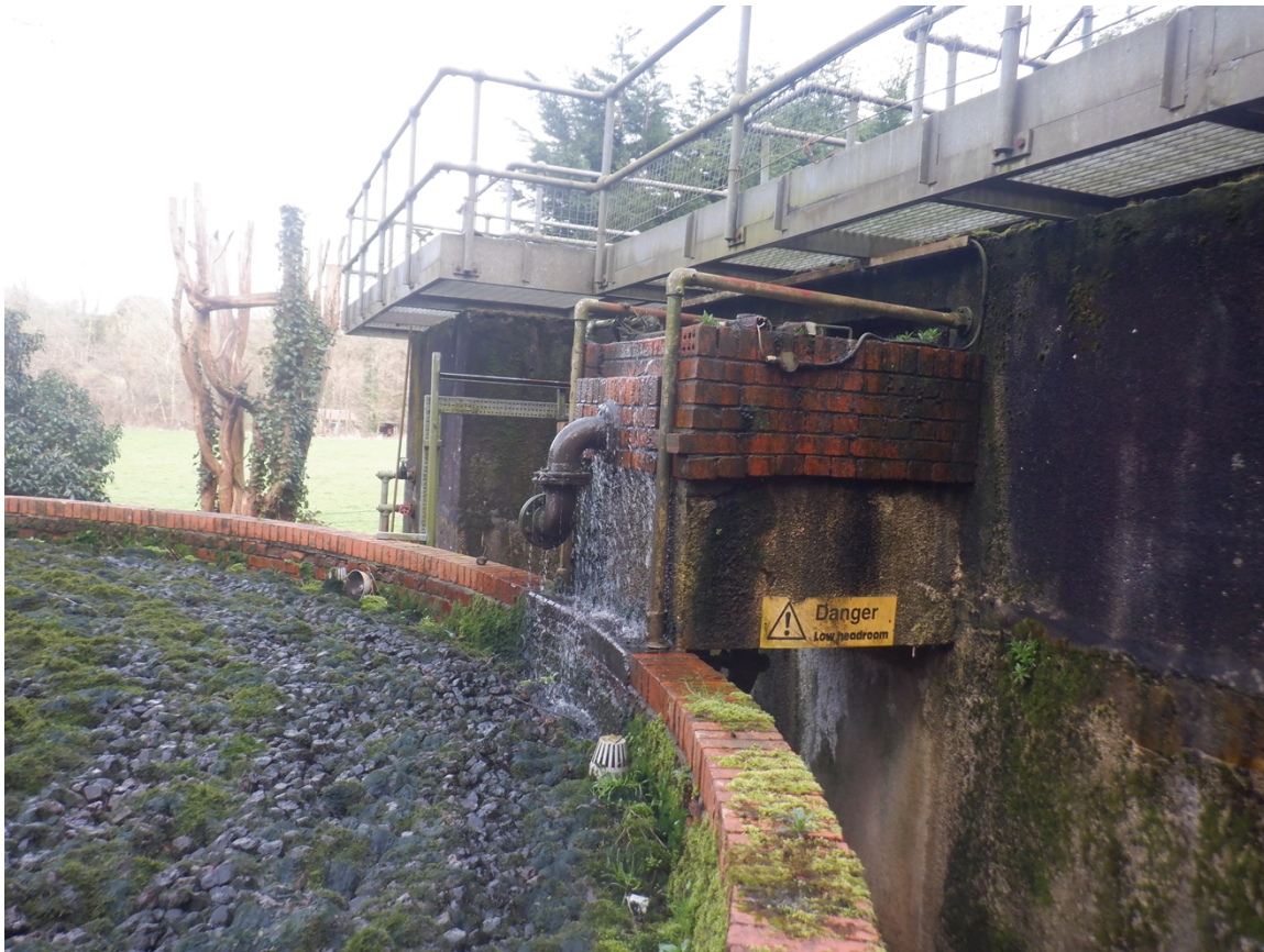
Photo showing chamber overflowing onto filter bed.
