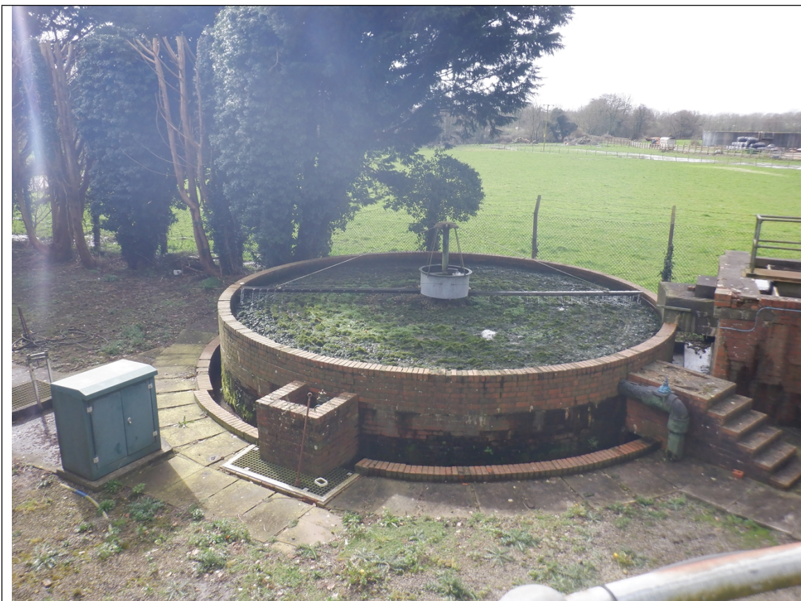
Photo showing filter bed.
