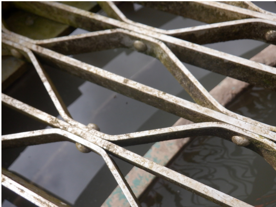
Photo showing submerged baffle in Primary Settlement Tank.
