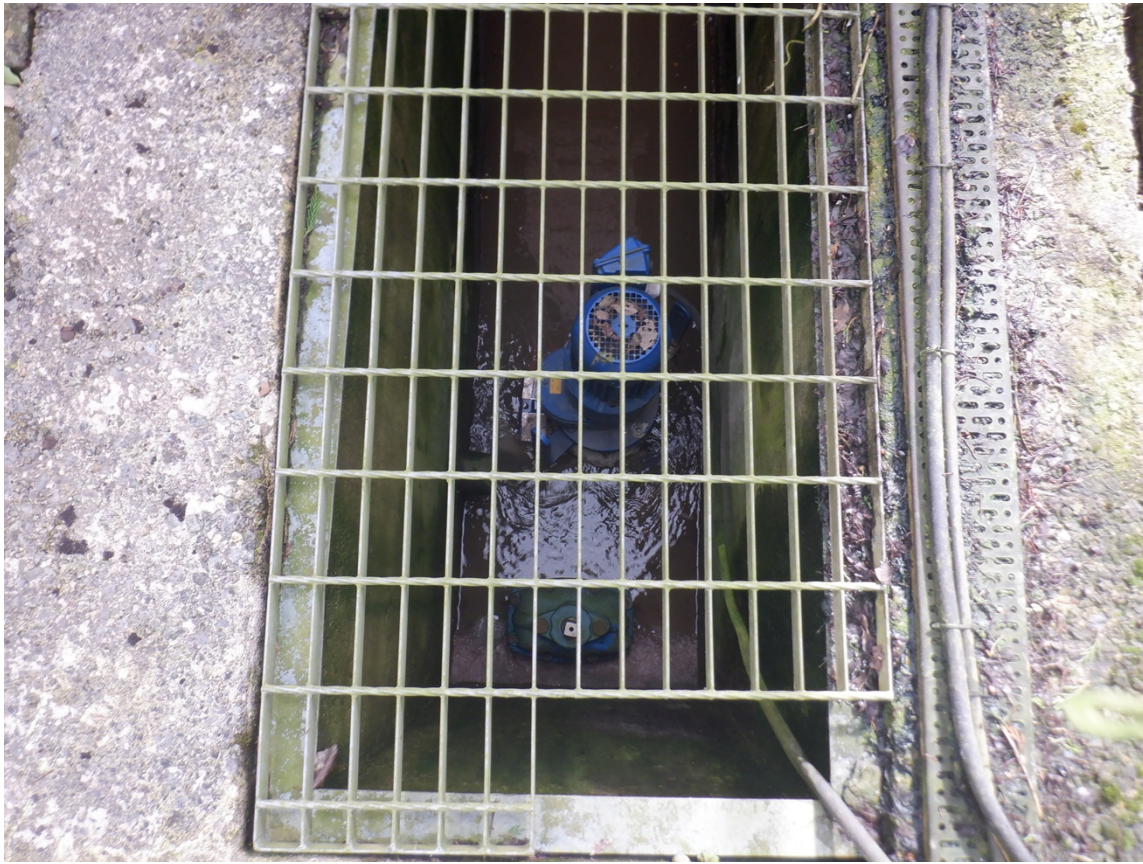
Photo showing macerator at inlet to Bancyfelin WWTW.
