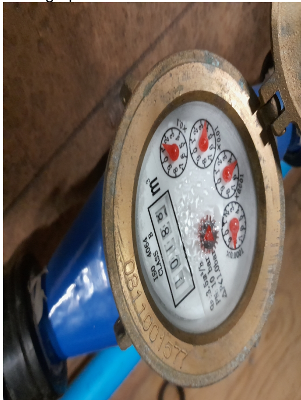
Photograph 1 – Meter at Visitor Centre
