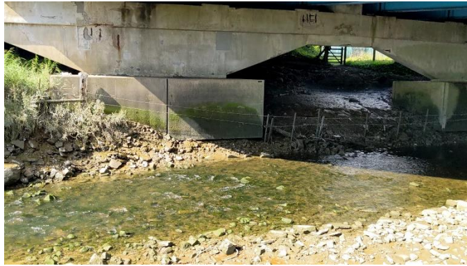
Photo 2: South west (downstream) concrete pier with protection panels. Undercutting of the concrete protection panel.
