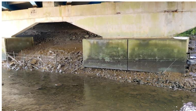
Photo 3: North west (upstream) concrete pier with protection panels. Undercutting of the concrete protection panel.
