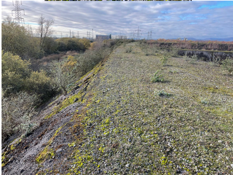
Plate 4-1 Tension Cracks on Surface of Embankment of Lagoon 27
