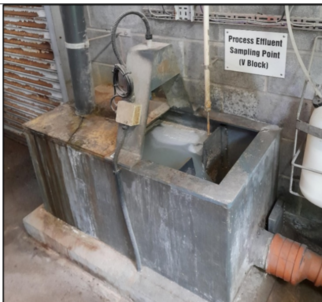
Image 2 – DAF showing effluent discharge housed within a unit
