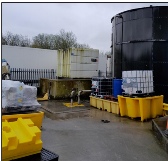
Image 1 – showing part of the effluent treatment plant with chemicals on secondary containment bunds
