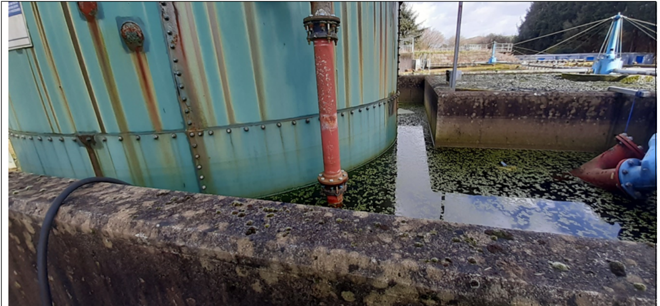
photo showing rainwater collected inside sludge holding tank bunded area.
