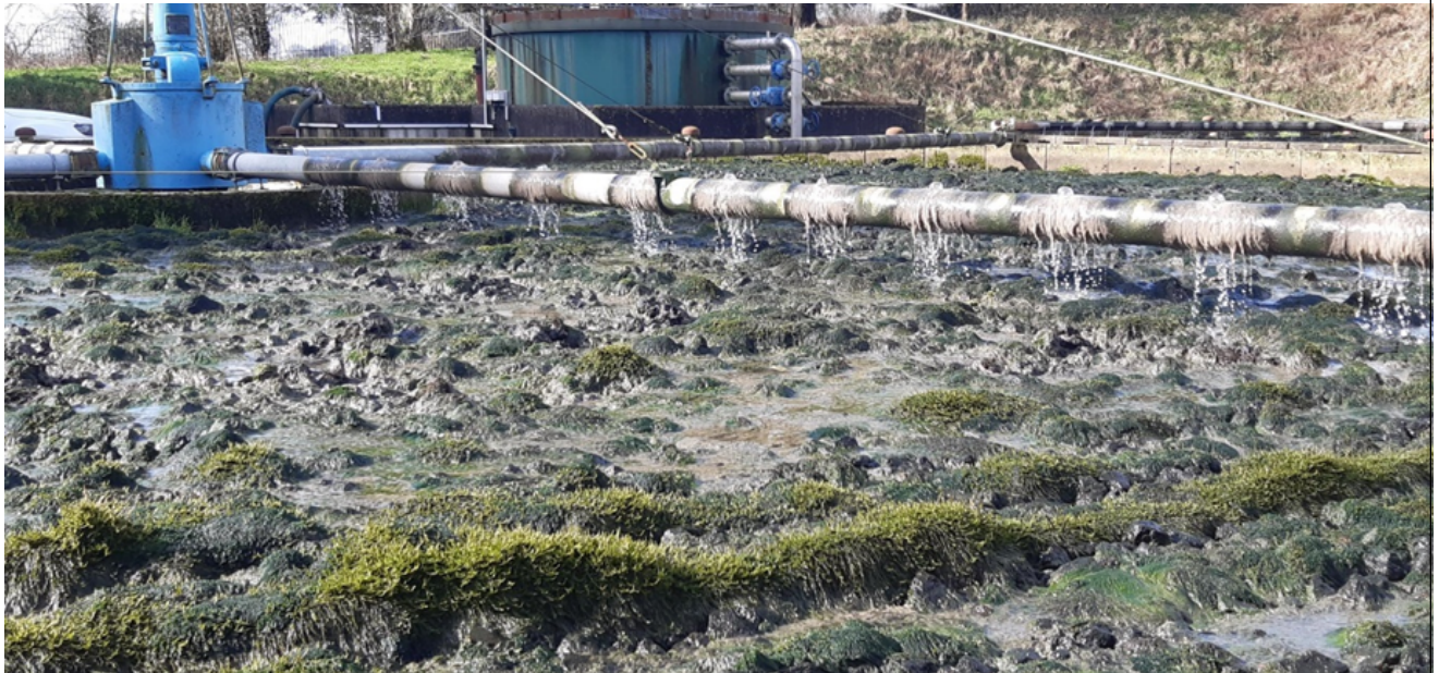
Photo showing build up of solids on filter bed.
