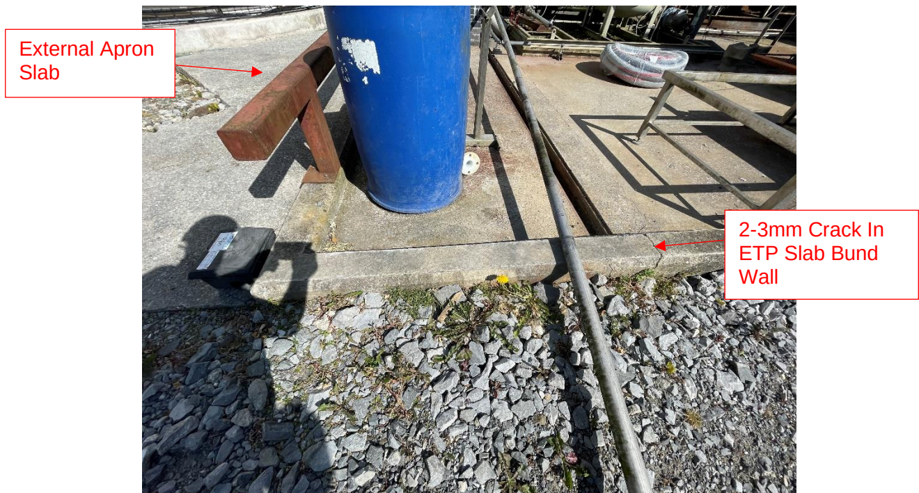
Photograph 6: Crack In Bund Wall
