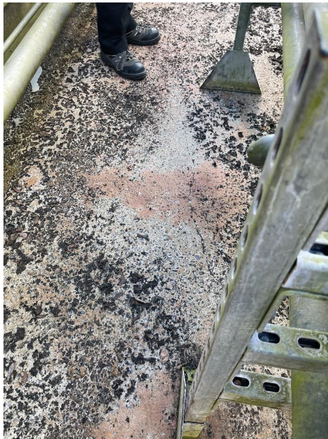
Photograph 20: 2-3mm Crack Propagating In Centre Of Main Slab
