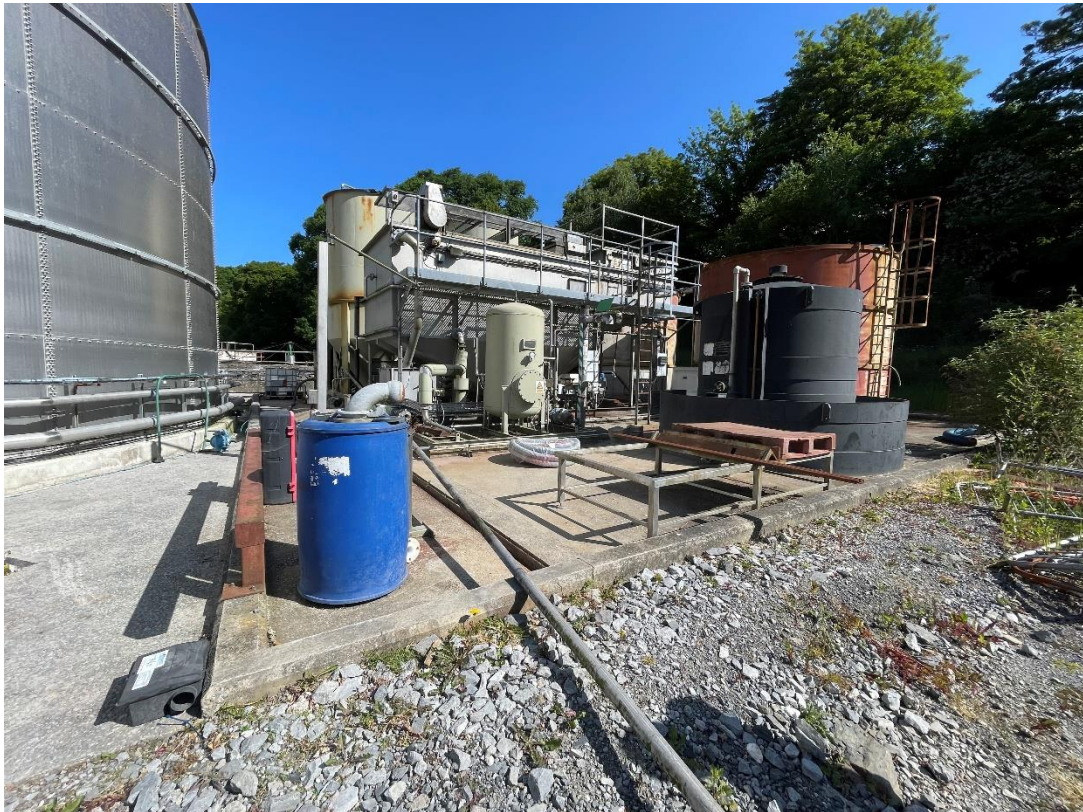
Photograph 3: Redundant ETP Process Plant – View 1
