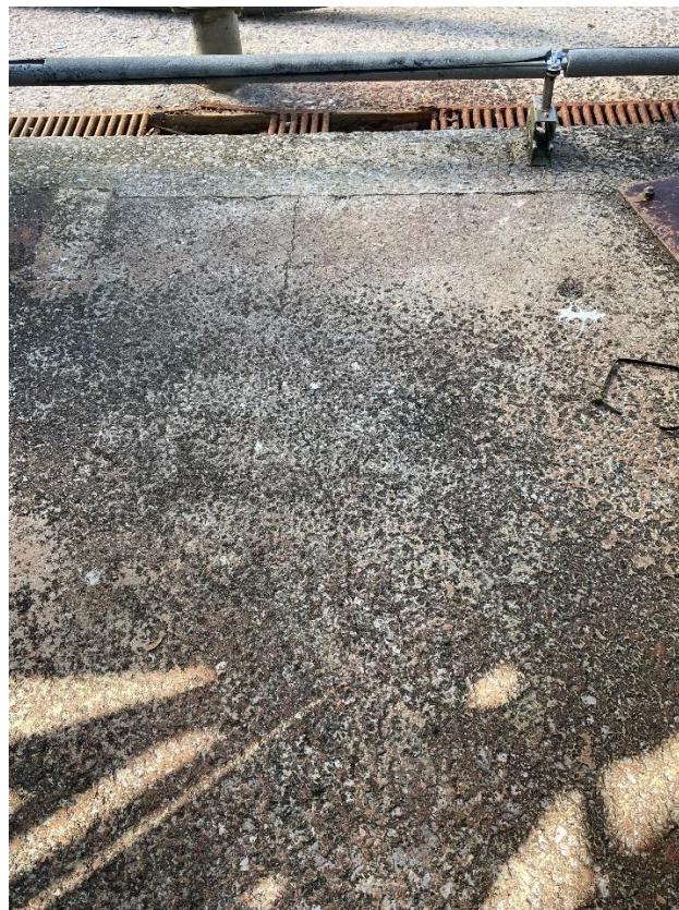
Photograph 12: 2-3mm Crack In Slab Adjacent To South Drainage Channel
