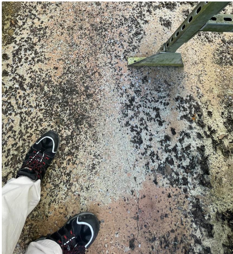
Photograph 22: 2-3mm Crack Propagating In Main Slab Between Equipment Supports
