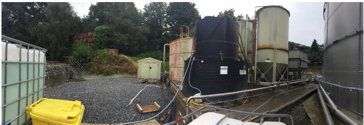
Photograph 4: Redundant ETP Process Plant – View 2
