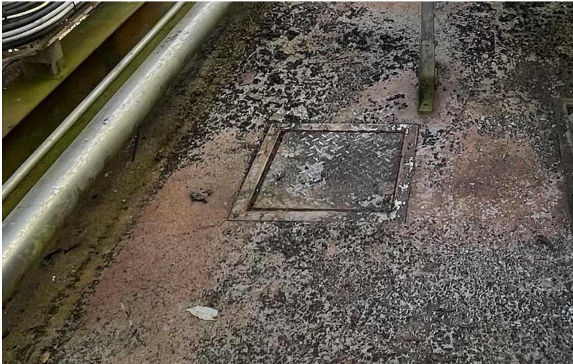
Photograph 19: 2mm Crack Propagating From Corner of Valve Chamber
