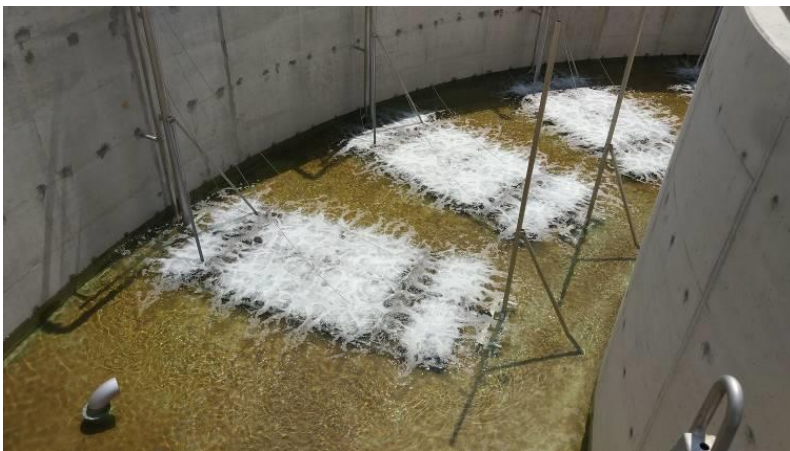
Aeration grids during start-up
