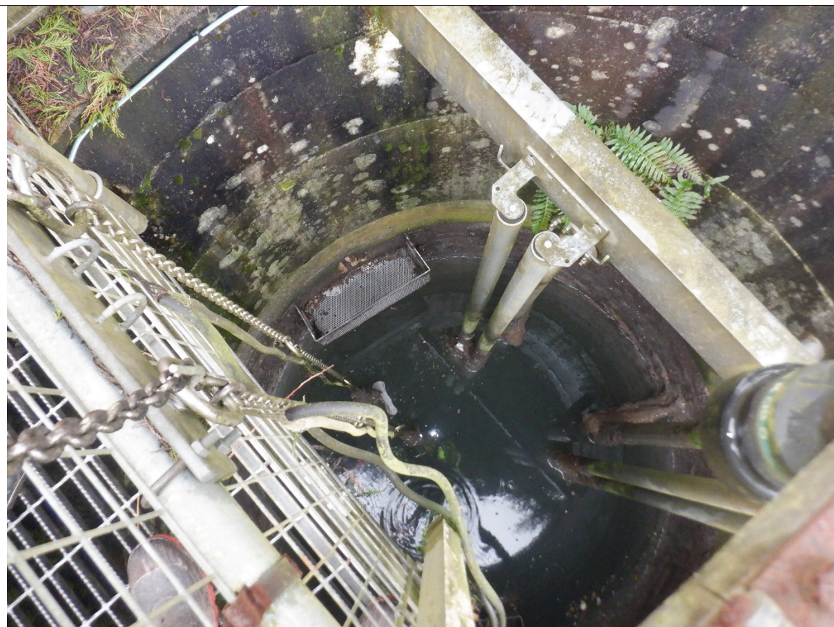
Figure 1 Storm tank with screen
