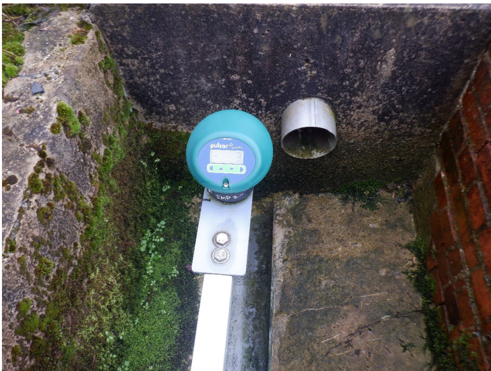
Figure 1: Storm overflow pipe on the inlet with EDM flow monitor.
