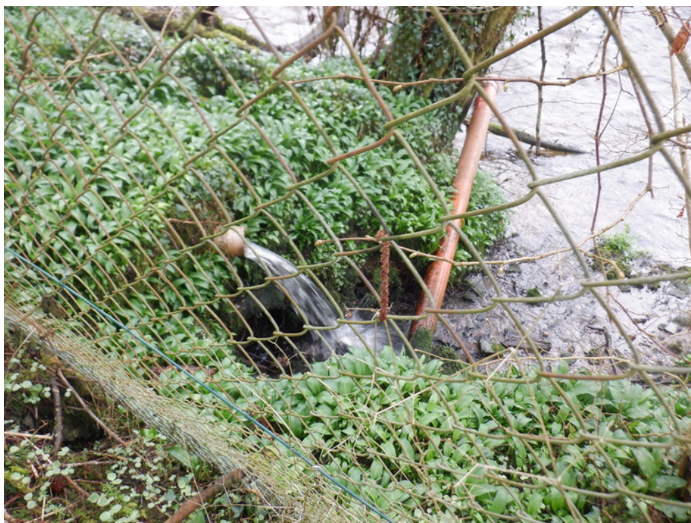
Figure 3 Discharge pipe for the storm was snapped as seen on the right.
