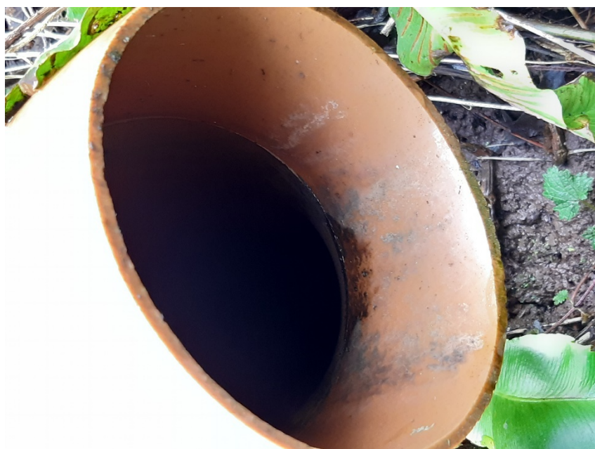
Figure 4: Discharge pipe showing staining
