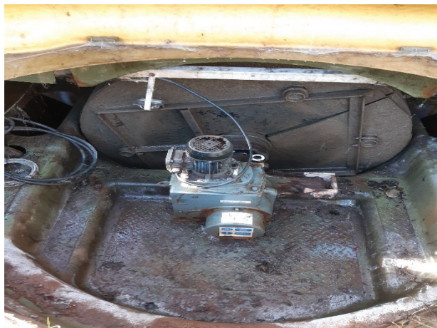
Figure 4 Final chamber of the system
