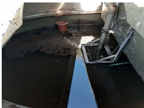
Figure 2 First chamber of system with scum
