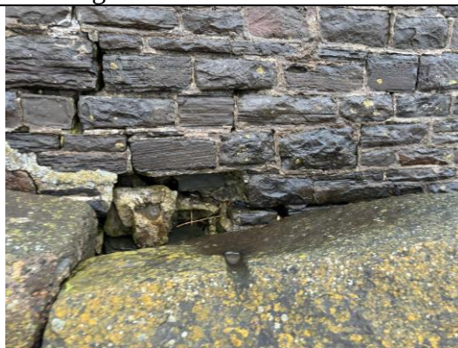
Void low level of wall
