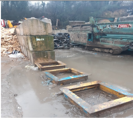
Figure 2: External view of interceptor system
