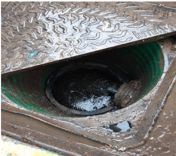
Figure 3: First interceptor chamber
