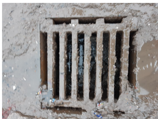
Figure 1: Manhole chamber in yard feeding into interceptor
