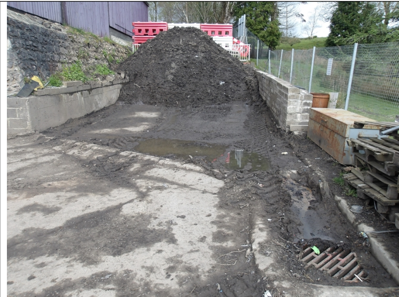
(De-watering waste blocking drainage channel)
