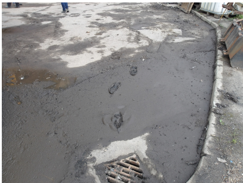
(Build of waste around drain)
