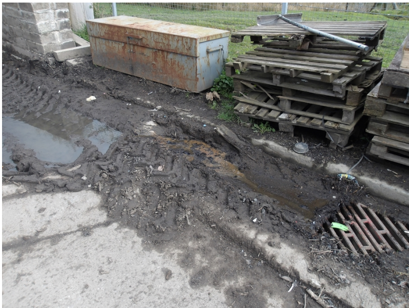
(De-watering waste blocking drainage channel)
