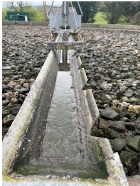
Image 5, final effluent sampling point
