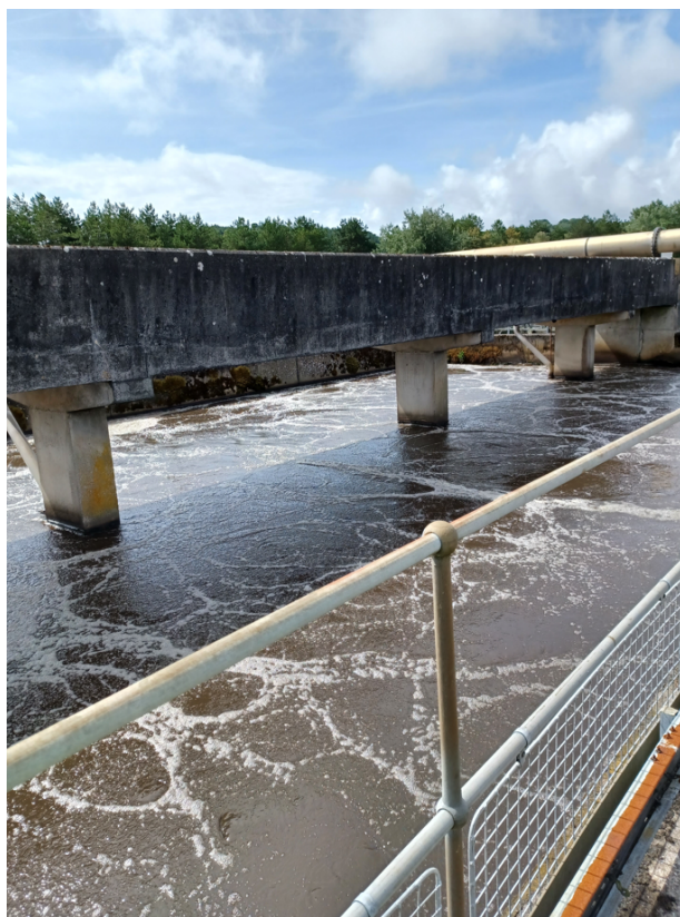
Picture 3: fully functioning aeration chamber
