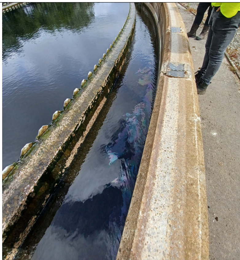
Picture 5: Final effluent tank no.4 with oil visible on surface
