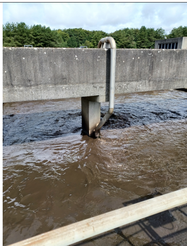
Picture 4: Aeration chamber with faulty aerator
