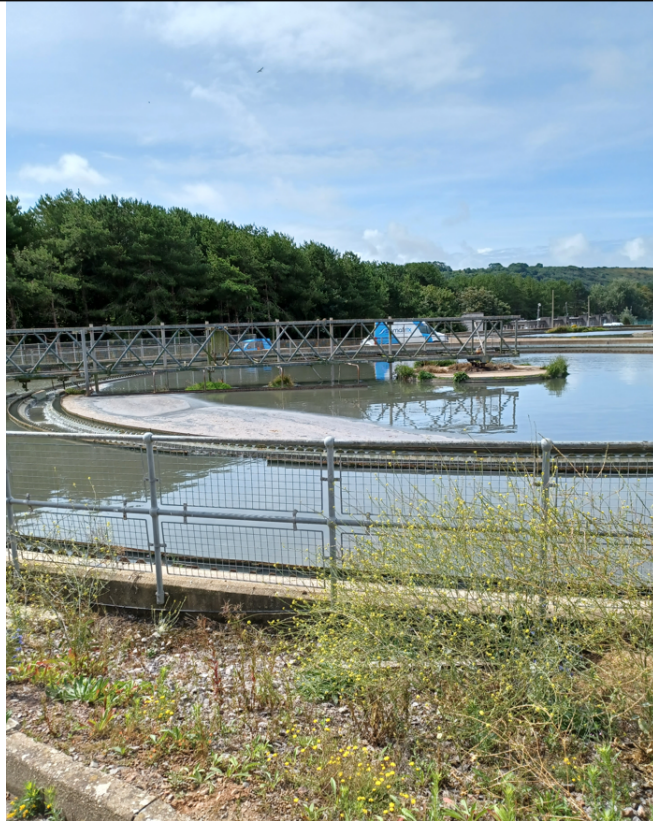
Picture 2: Primary settlement tank
