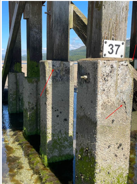
Various spilled concrete
