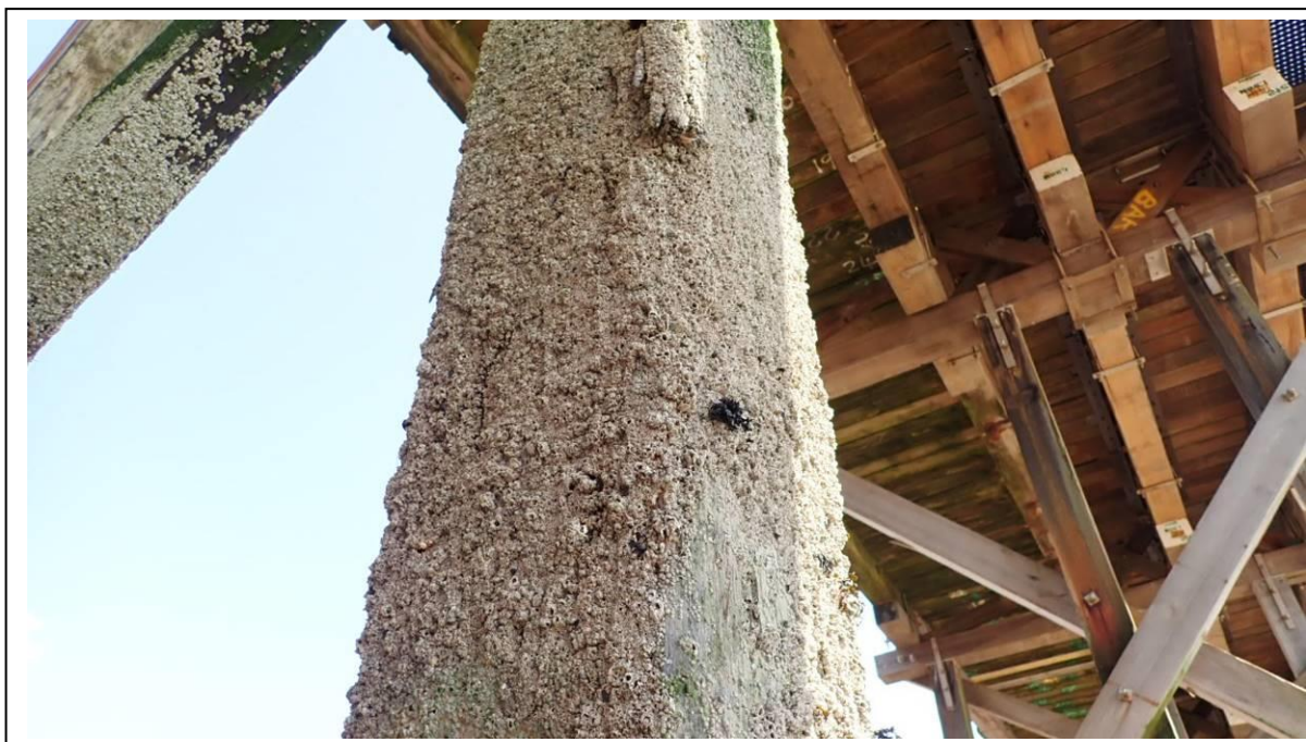
Photo 38 Trestle 109 – Pile 3, Splinter to DS HM corner
