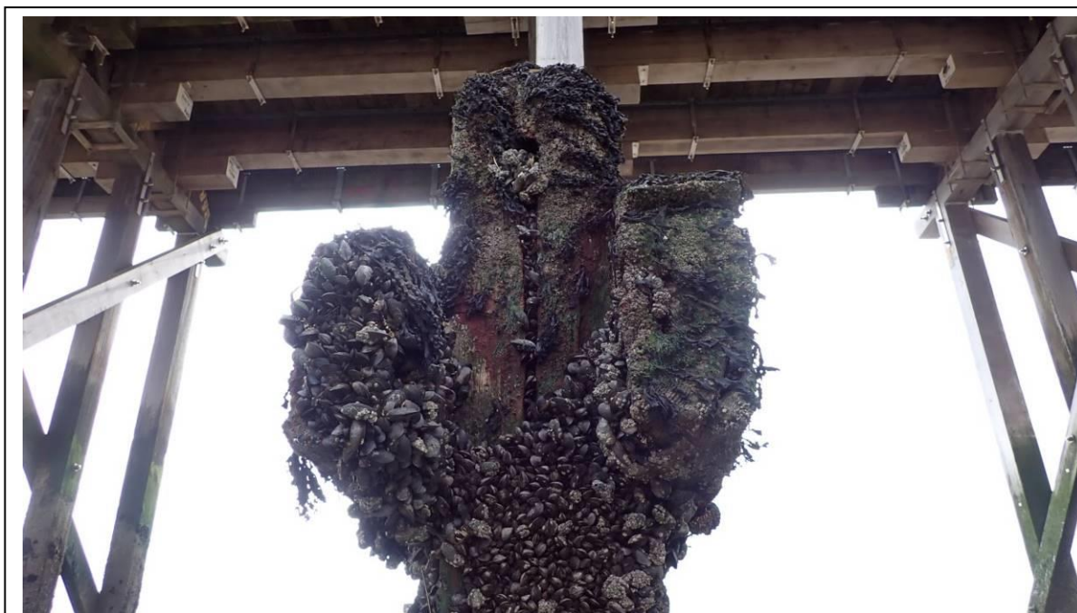
Photo 54 Trestle 82 – Upside outrigger, split
