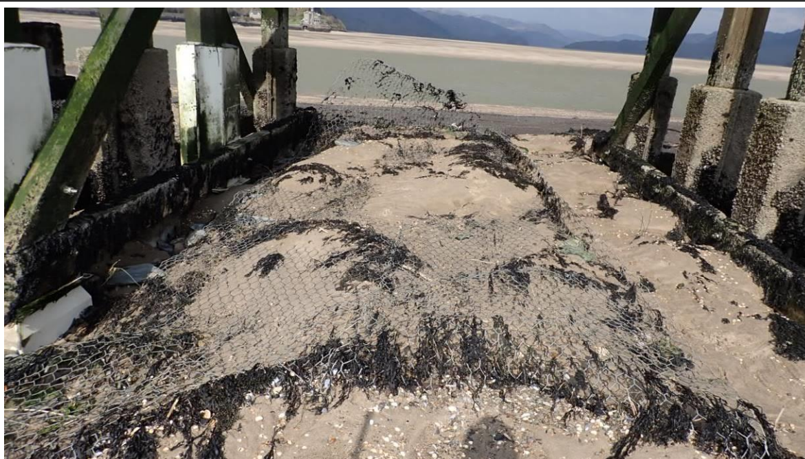
Photo 57 Typical mesh on bed – poor condition, lifting to span 1 - 80
