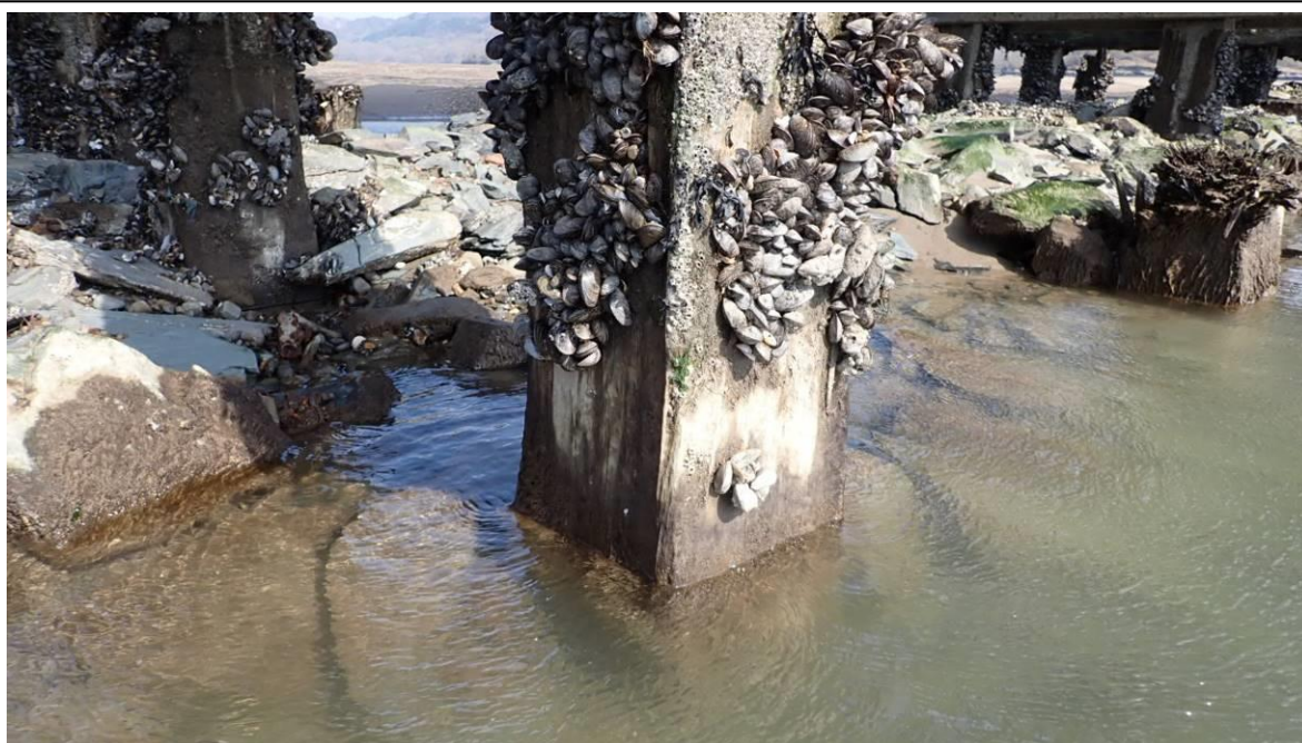
Photo 41 Trestle 98 – Pile 1, splits and thinning
