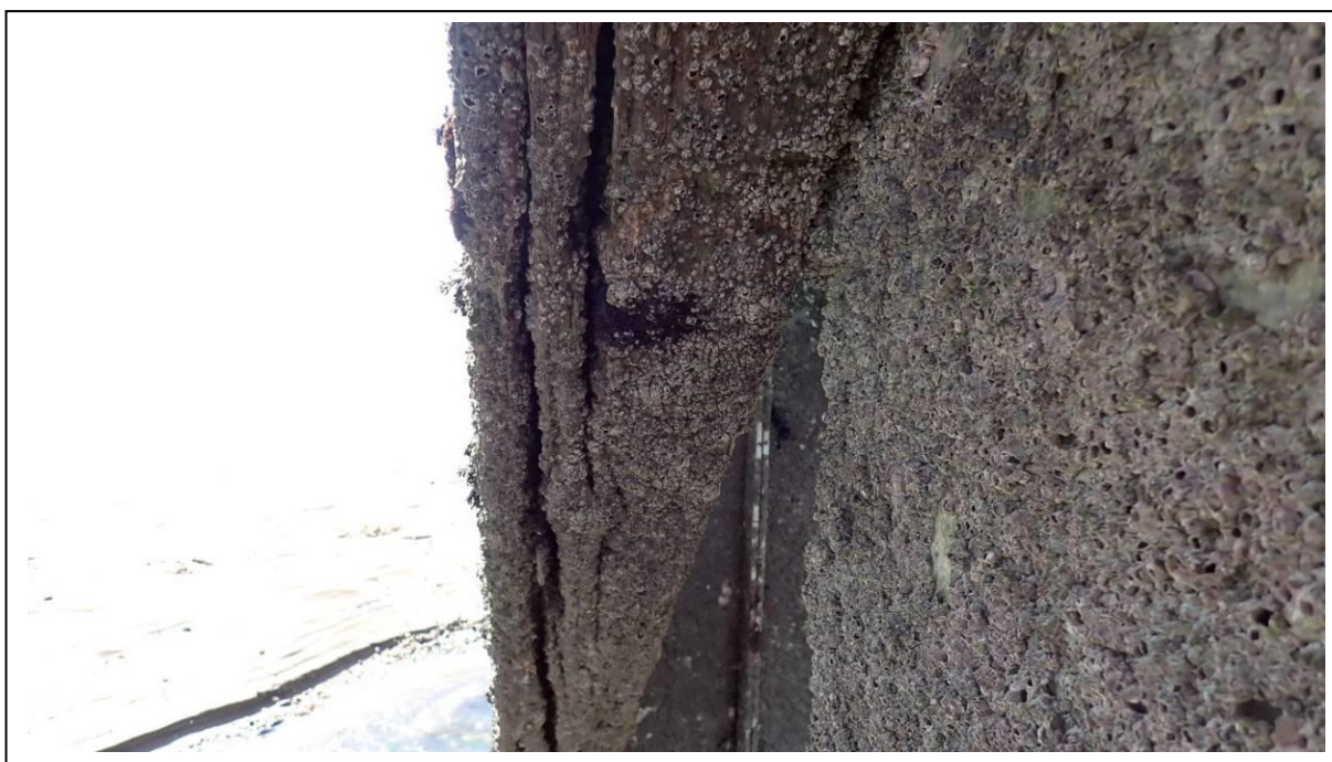
Photo 32 Trestle 33 – LM diagonal brace has low level splits
