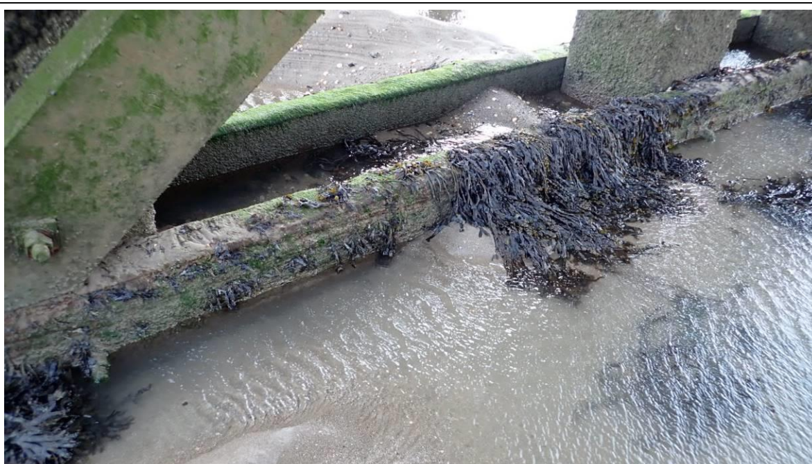
Photo 16 Trestle 16 – HM horizontal brace, splits and minor decay
