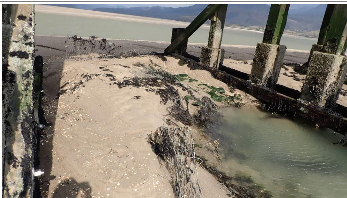
Photo 58 Typical view of damaged mesh
