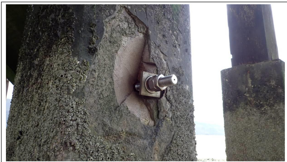
Photo 45 Trestle 51 – Pile 2, spalling at bolt [NEW]
