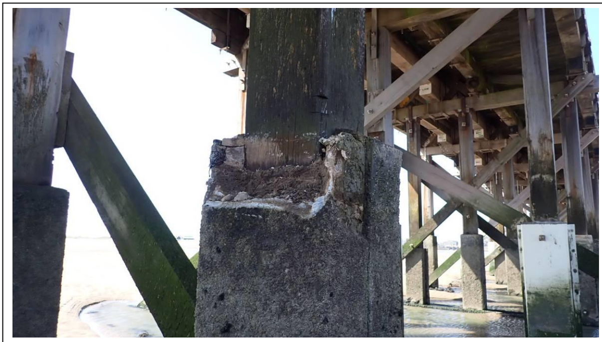
Photo 31 Trestle 31 – Pile 4, loss of casement at top, LM face [NEW]
