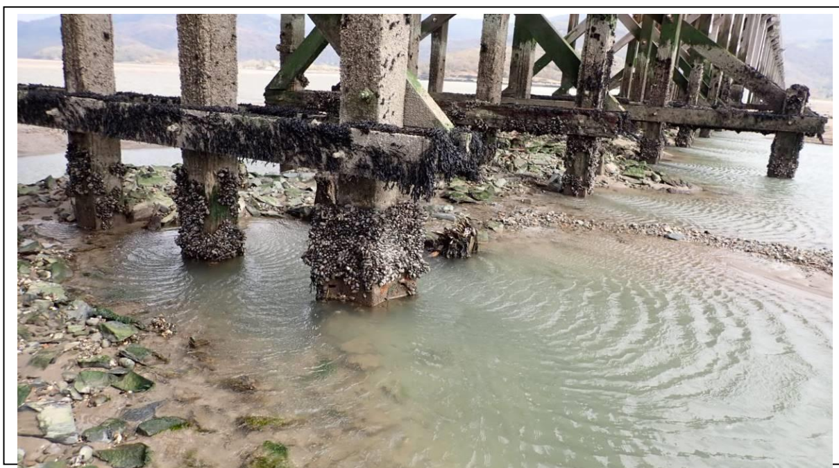
Photo 52 Trestles 74 – 80 & 84. Typical scour pools forming
