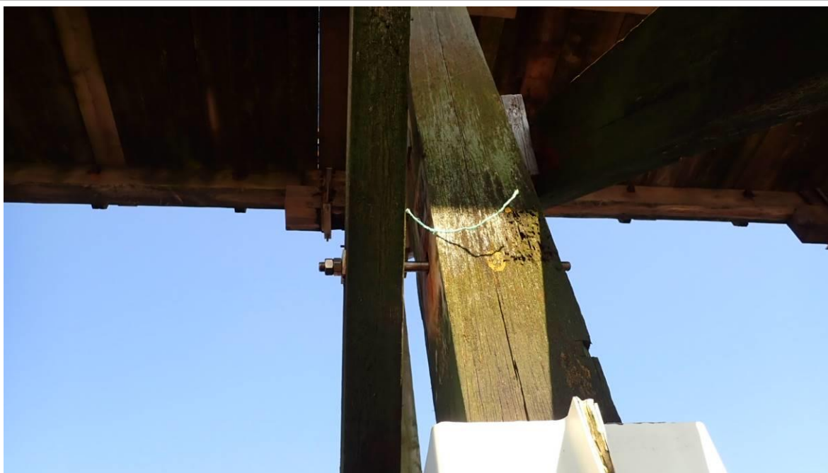
Photo 35 Trestle 48 – Pile 3, missing packer to HM Diagonal brace
