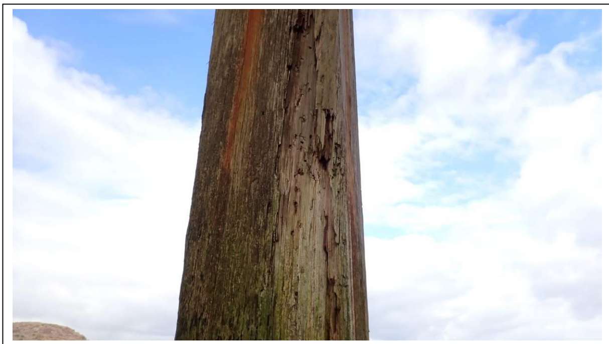
Photo 9 Trestle 2 – Pile 4, decay
