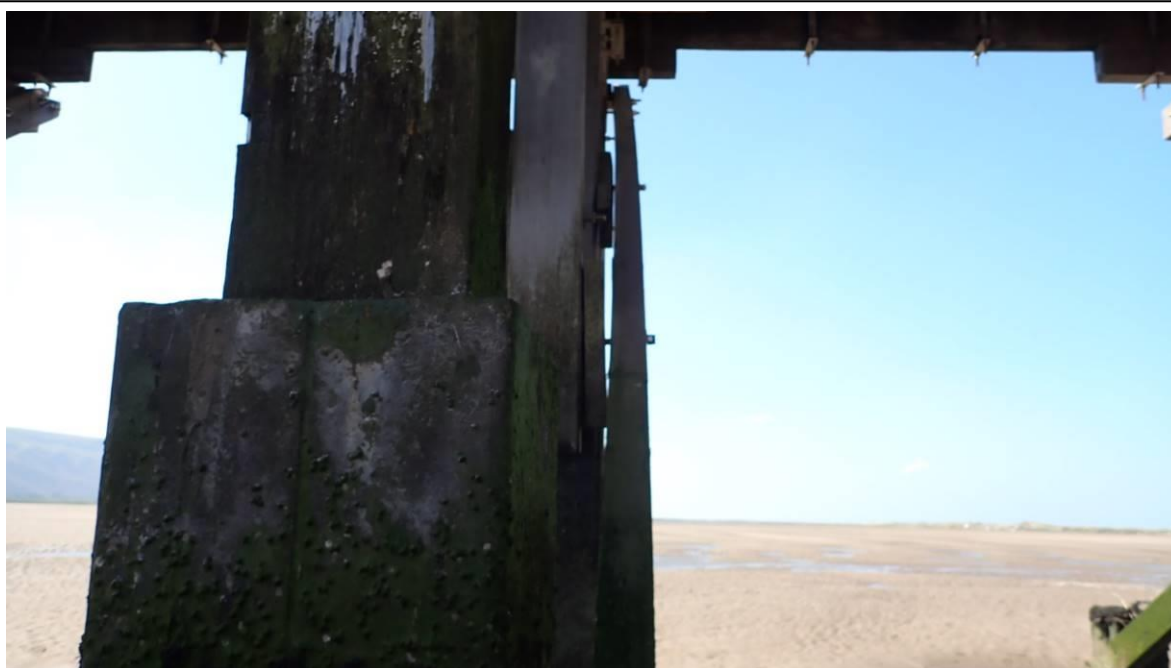
Photo 15 Trestle 16 – New HM diagonal brace is bowed.
