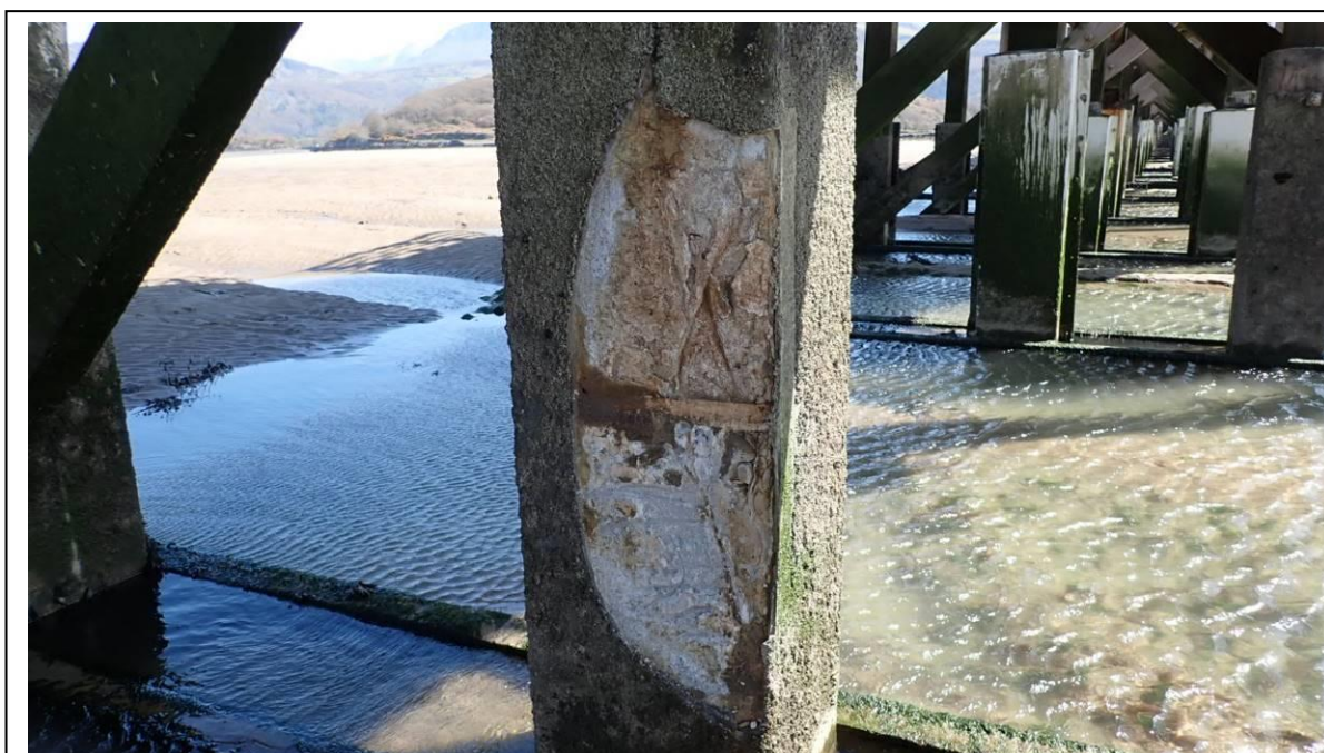
Photo 30 Trestle 31 – Pile 3, NEW area of spalling to encasement.
