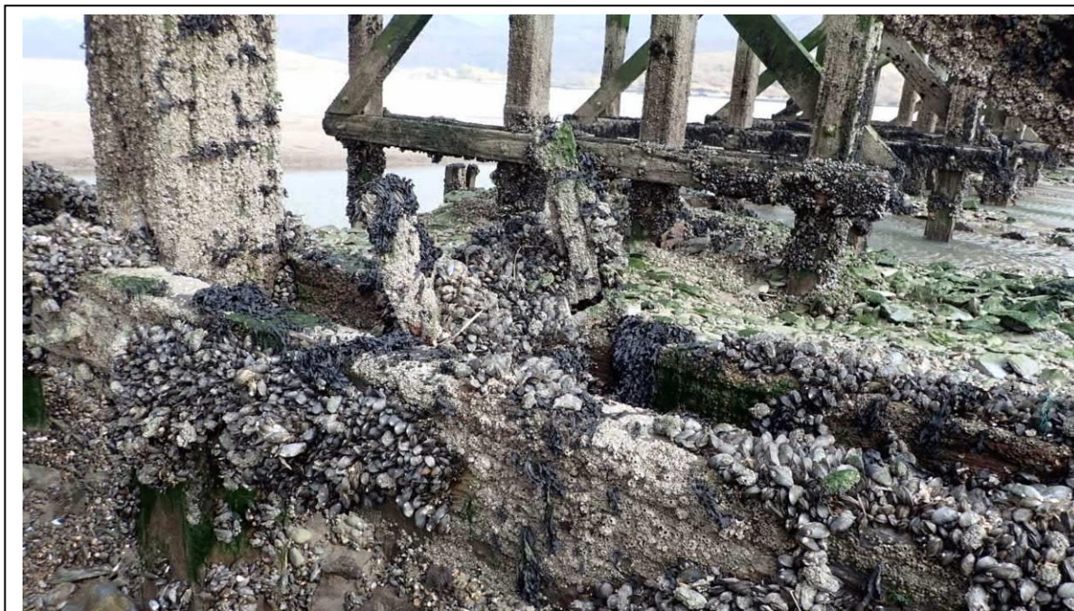
Photo 53 Trestle 82 – Down side outrigger, broken between horizontal and diagonal brace
