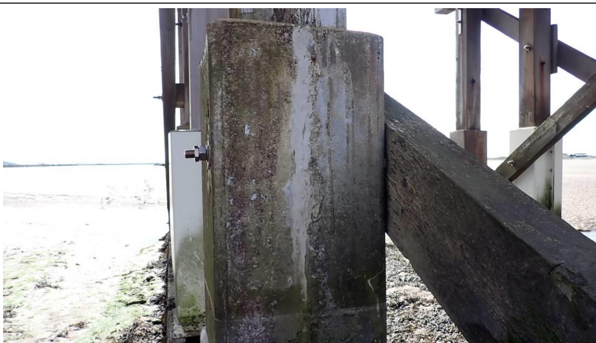
Photo 8 Trestle 2 – Pile 4, area of repair
