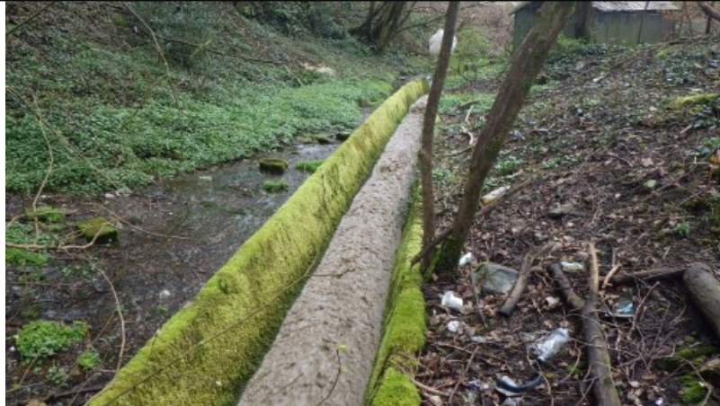
Figure 5 – Site visit photos: Downstream view of silty water seen running within the concrete channel at ST2194295860.
