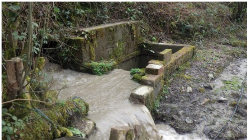
Figure 23 – Site visit photos: Silted water was seen entering the open culvert at ST2245896470. No samples were taken due to access and H&S concerns at the time of the visit.
