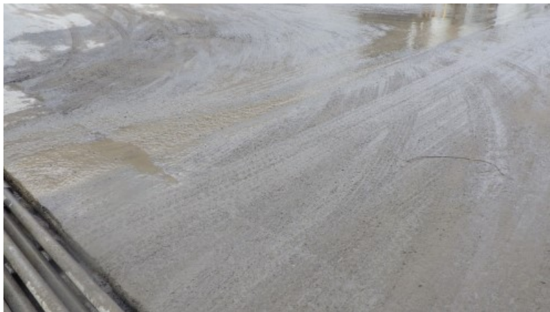
Figure 12 – Site visit photos: Quarry road runoff seen entering the catch pit at ST2223896331.
