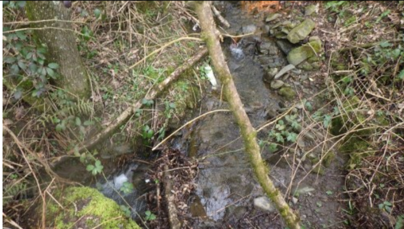
Figure 22 – Site visit photos: Nant Hafod-fach directly upstream of where it is culverted beneath the site at ST2245396500 as observed during the visit. No visible pollution present.
