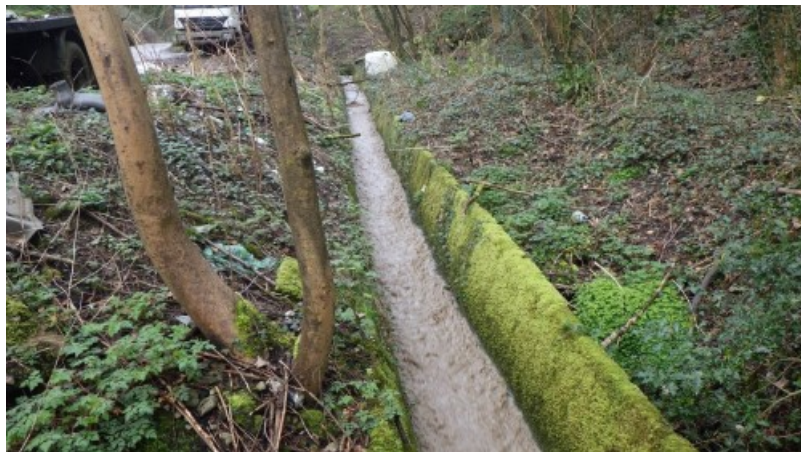
Figure 6 – Site visit photos: Upstream view of silty water seen running within the concrete channel at ST2194295860.
