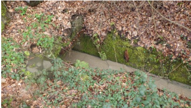
Figure 14 – Site visit photos: The silty discharge observed leaving site and discharging into the concrete channel at ST2223596317.
