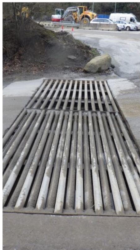
Figure 13 – Site visit photos: The catchpit as observed during the visit at ST2223896331. Appears to be working as designed. No concerns noted.
