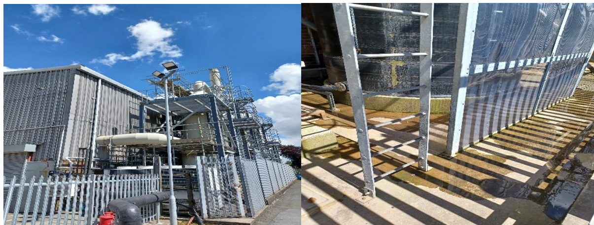
2x Scrubber units shown on left and leaking liquid from tank shown on right
