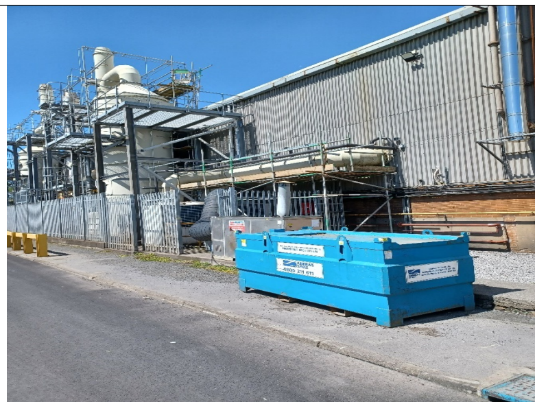
Temporary heating equipment and diesel storage bowser
