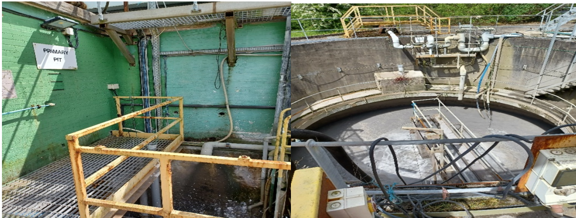
Effluent treatment plant stage 1 (left) Effluent treatment plant stage 2 (right)
