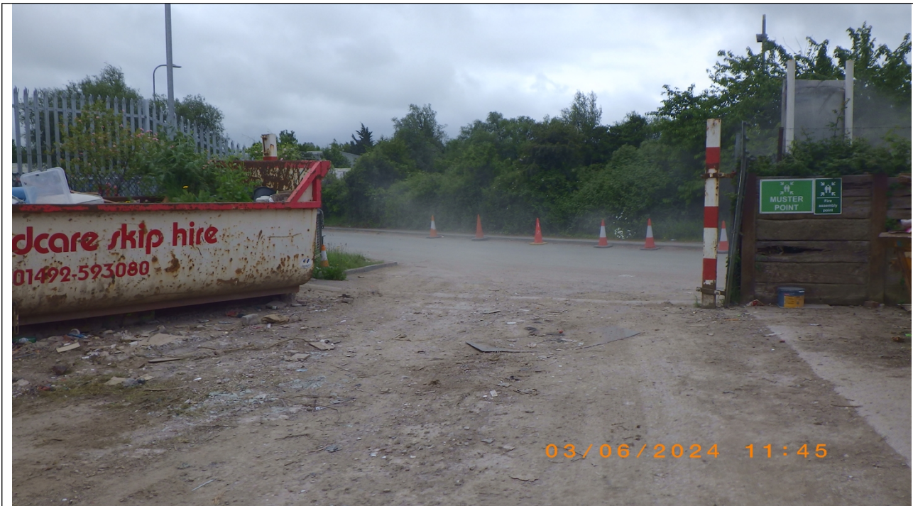
Photographs showing dust on site and dust emissions leaving site
