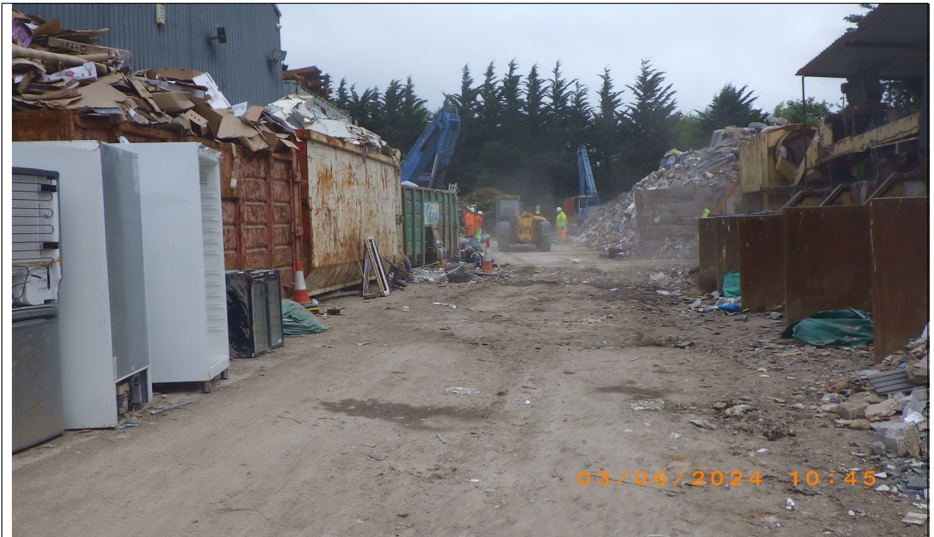
Photograph showing un made ground and dust generated from waste on site
