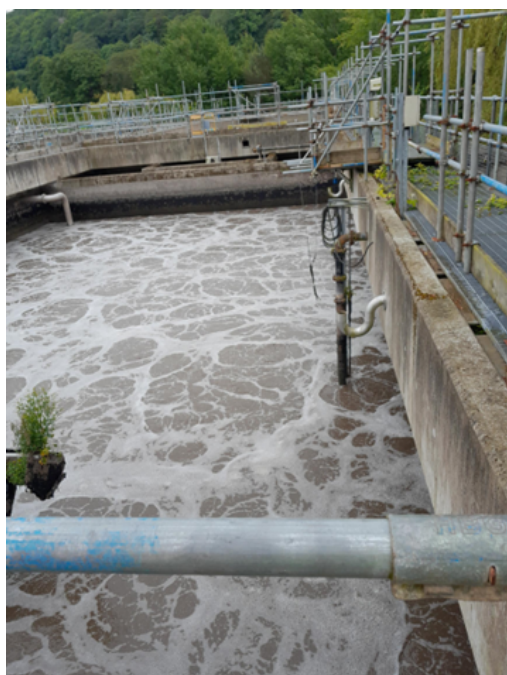
Image 4, SBR, Sequential batch reactor.
