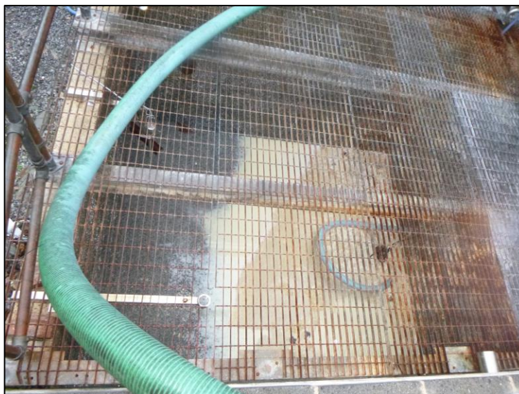
Image 2 - showing the sludge pit
