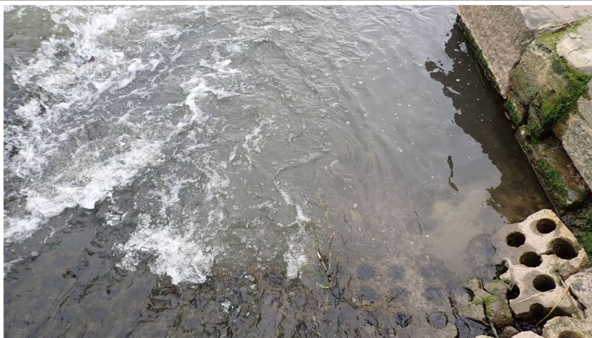
Photo 25 Area of missing invert –downstream high mileage
