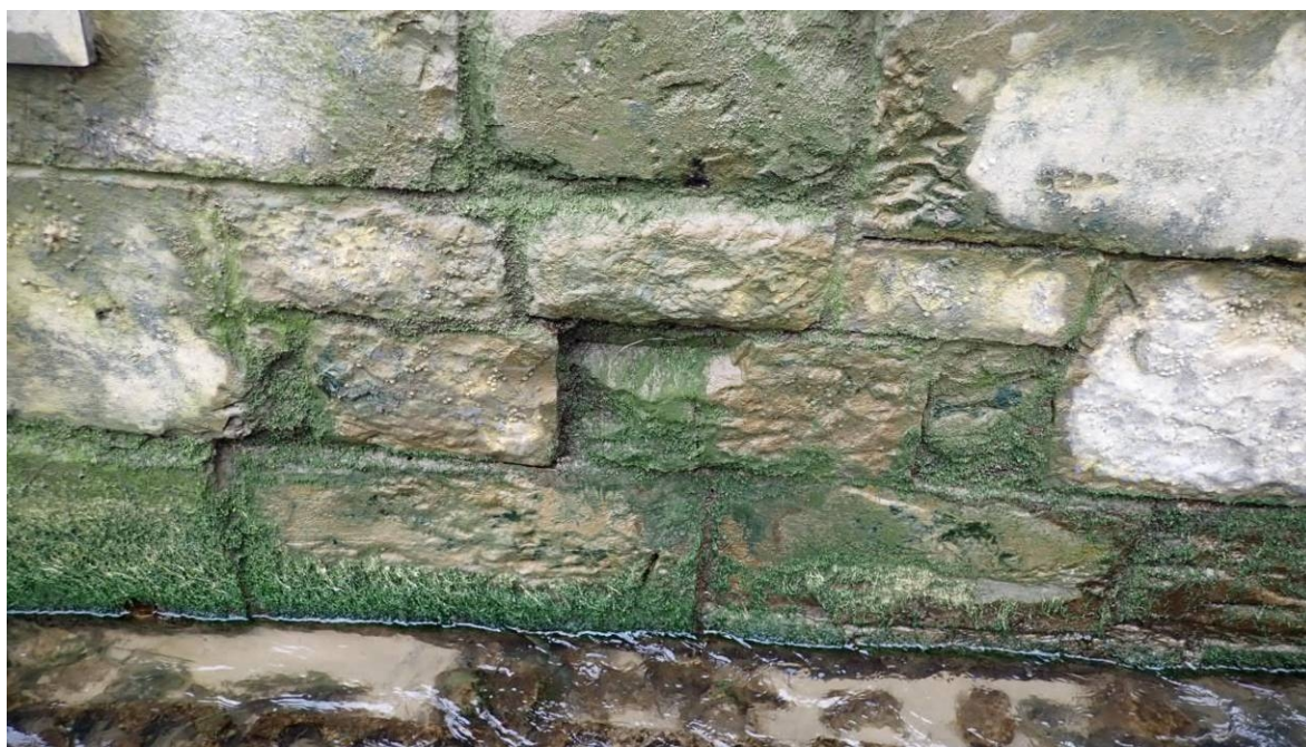
Photo 9 Area of spalling
