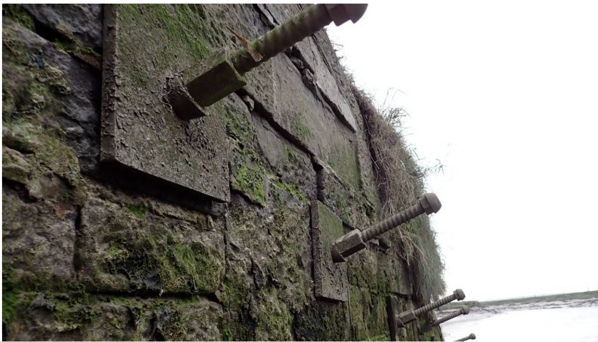
Photo 21 Bulge to wall
