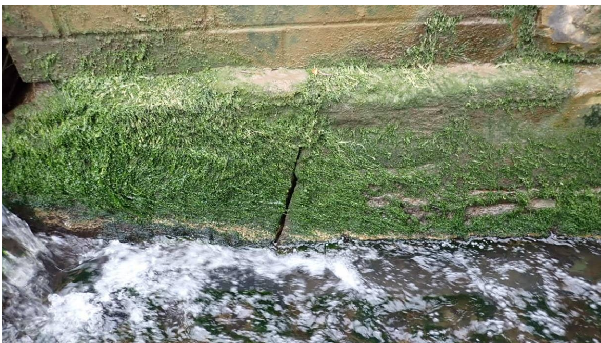
Photo 10 Through block fracture
