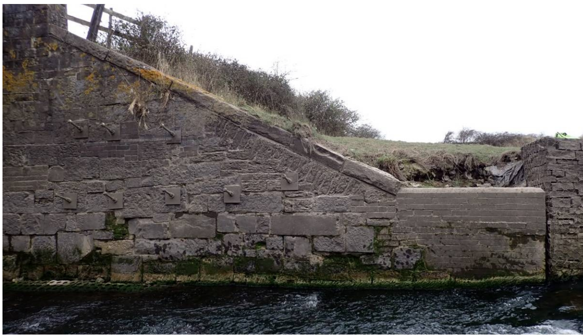
Photo 11 Upside high mileage wingwall
