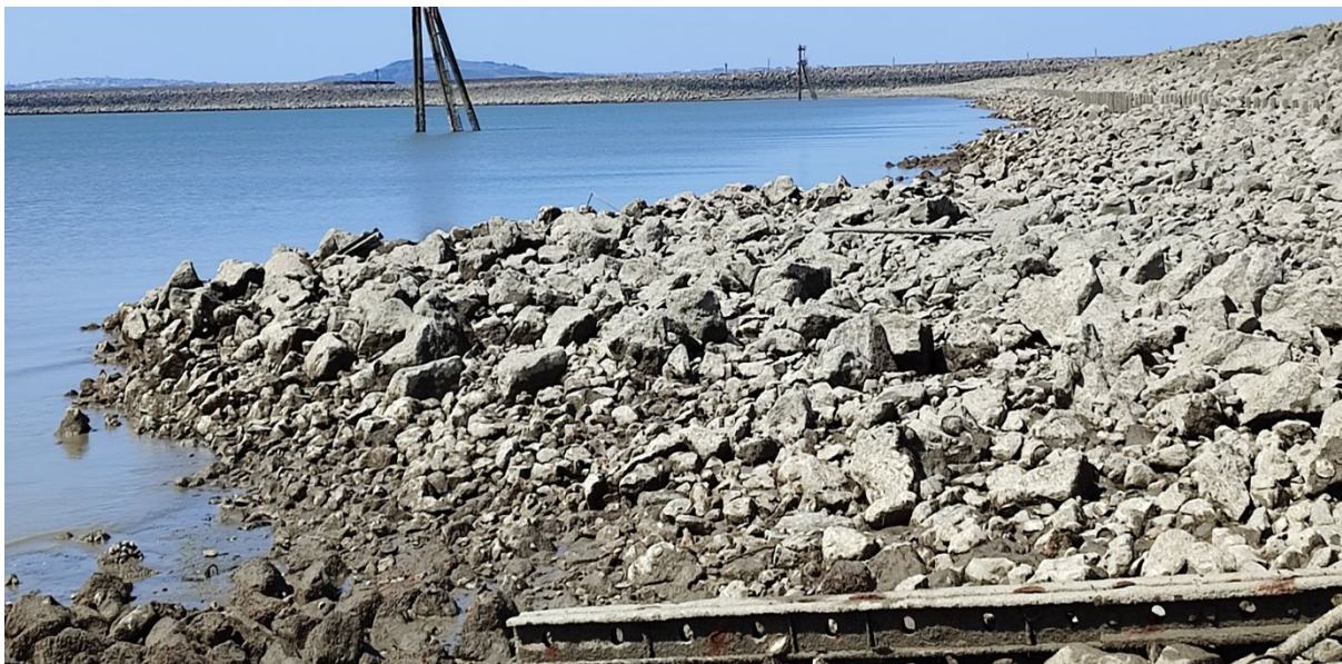
Image 7. Boulder sea defence with breakwater in distance
