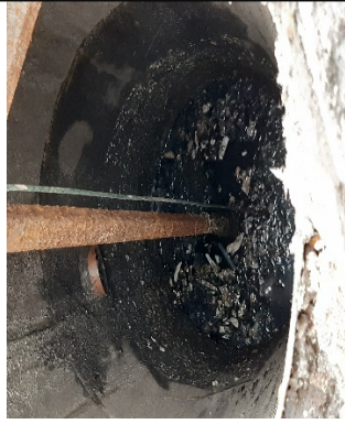
Figure 3: Final inspection chamber of interceptor
