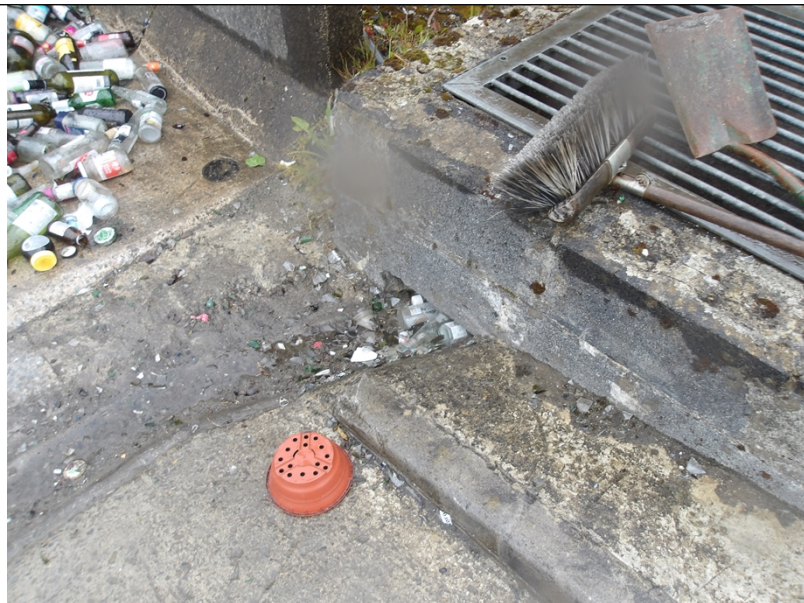
(Waste glass build up at entrance to drainage system)
