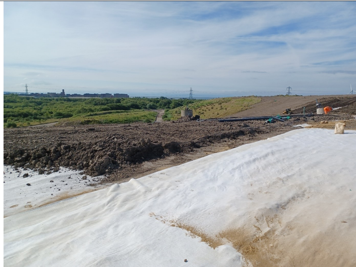
Photo above showing top of cell 16 which has been capped and restoration soils being laid on top.
