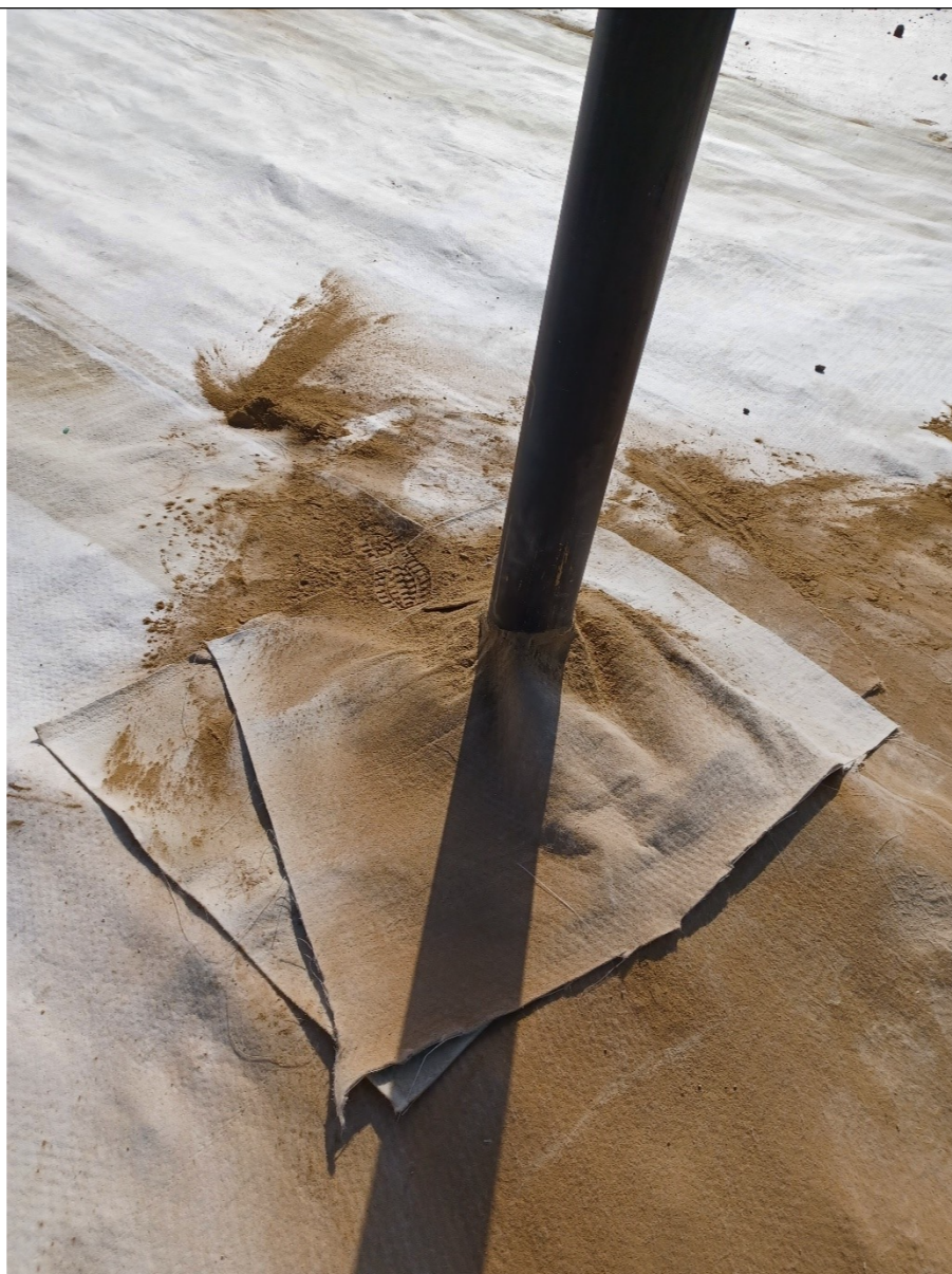
Photo above showing gas well on the top of cell 16 capped with Geological clay liner and coating of Bentonite powder.
