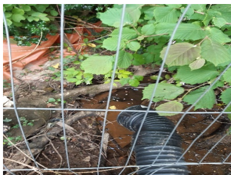
Figure 1: Discharge Point 1 showing no discharge
