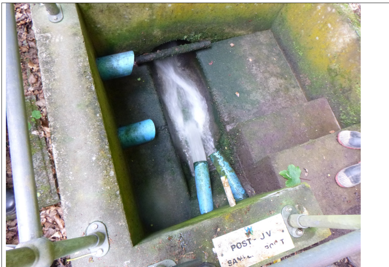
Figure 3 Final effluent point. 2 pipes on the left to be capped if they are not part of the permitted process.
