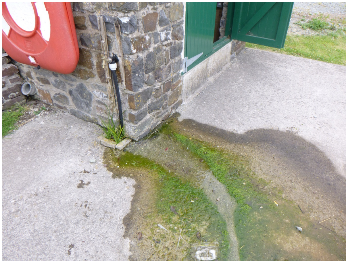
Figure 1. leak on the water supply tap outside, clean water, not sewage
