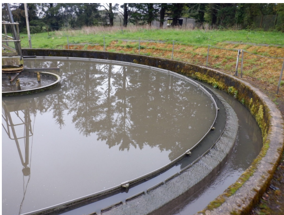
Figure 2 Storm settlement tank in old primary tank
