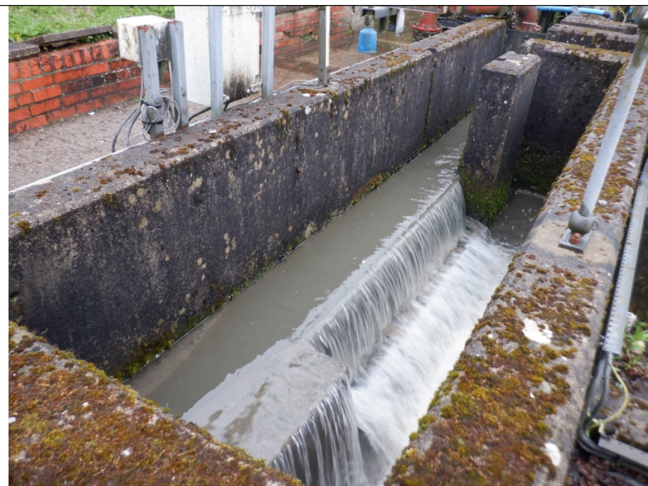
Figure 2: Storm overflow weir on inlet channel after the screen. Flows were over the height of the weir at the time of site inspection. EDM monitor is visible in the centre of the photo.
