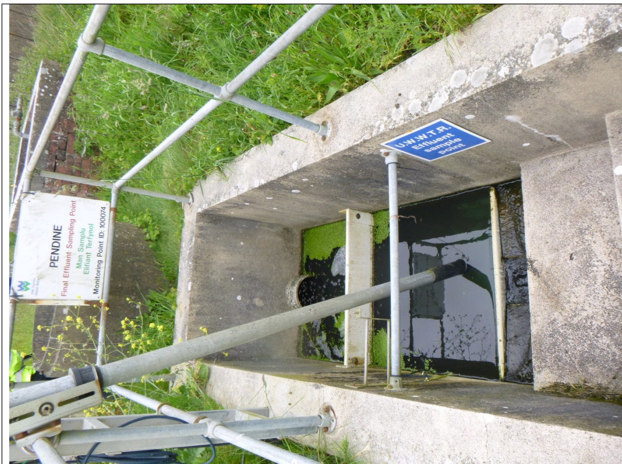
Final effluent sampling point
