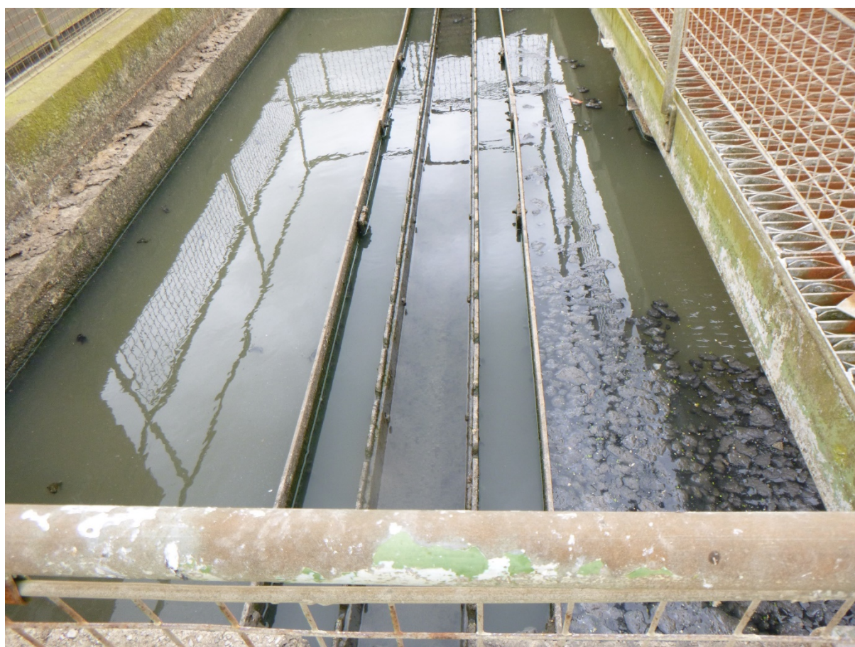
Primary settlement tank
