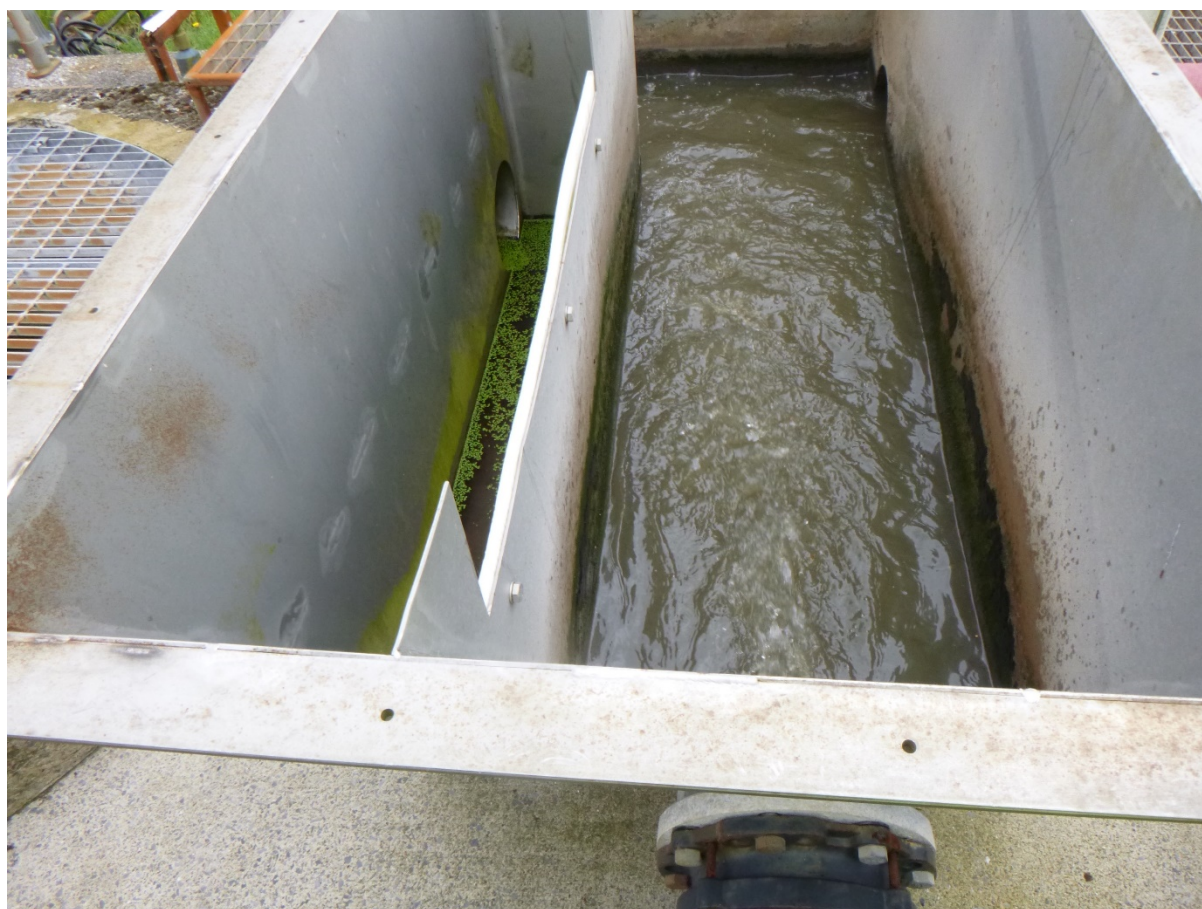
Figure 1 Inlet to works with Overflow weir for storm.
