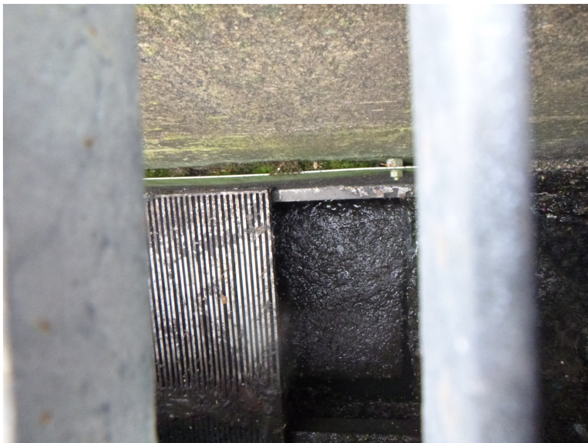
Figure 1 Bar screen on storm discharge
