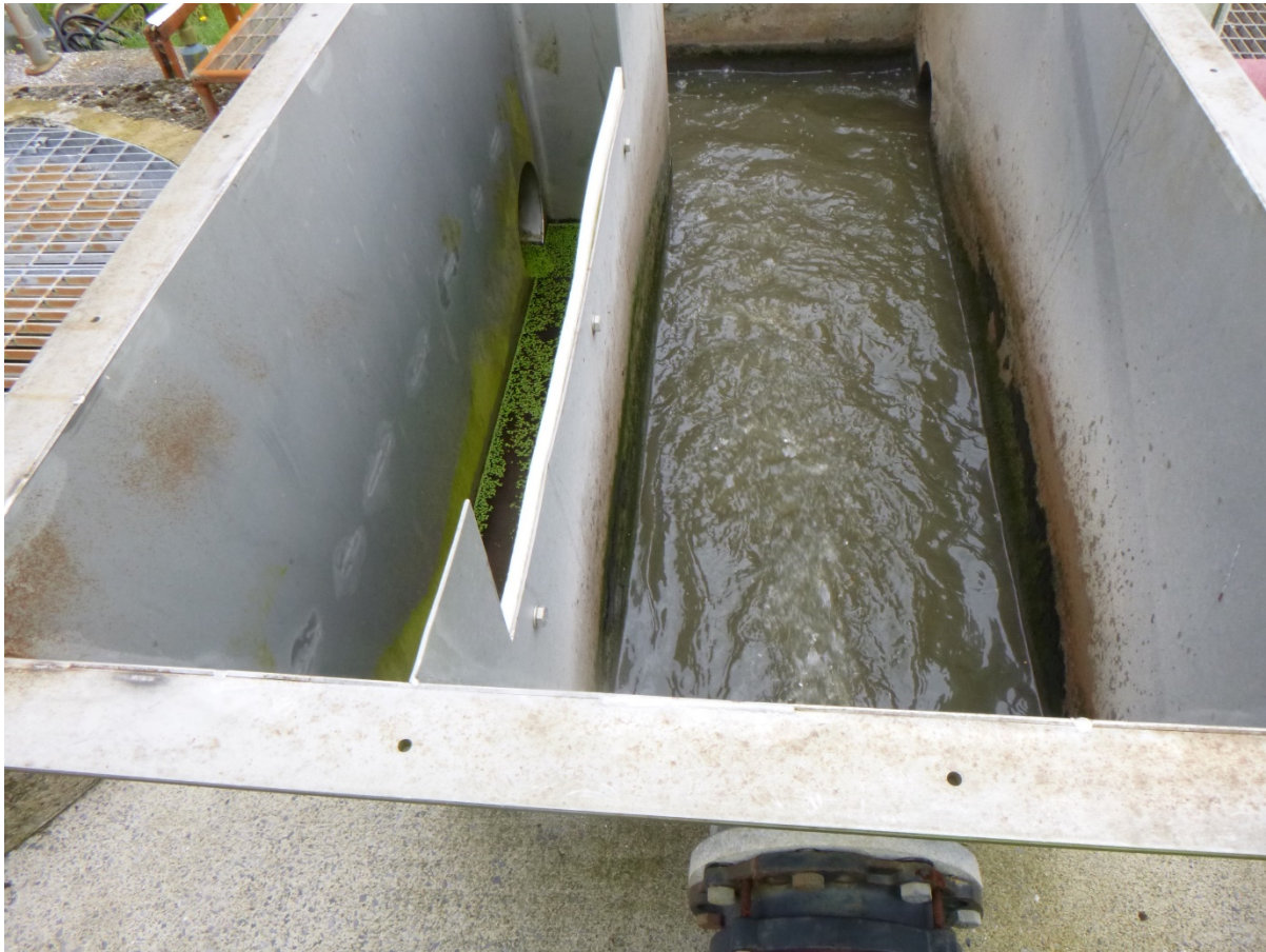
Figure 1- Inlet with storm overflow Weir and discharge point on the left of the photo. Flows were well below the height of the weir at the time of the inspection.
