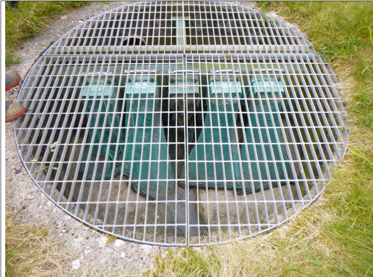
Figure 2- Storm flows are screen via sacks. These are emptied manually when full.
