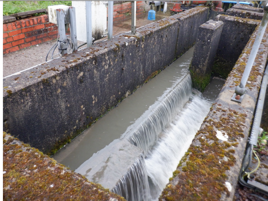
Figure 2: Storm overflow to storm tank after the screen, spilling to storm at the time of the visit.
