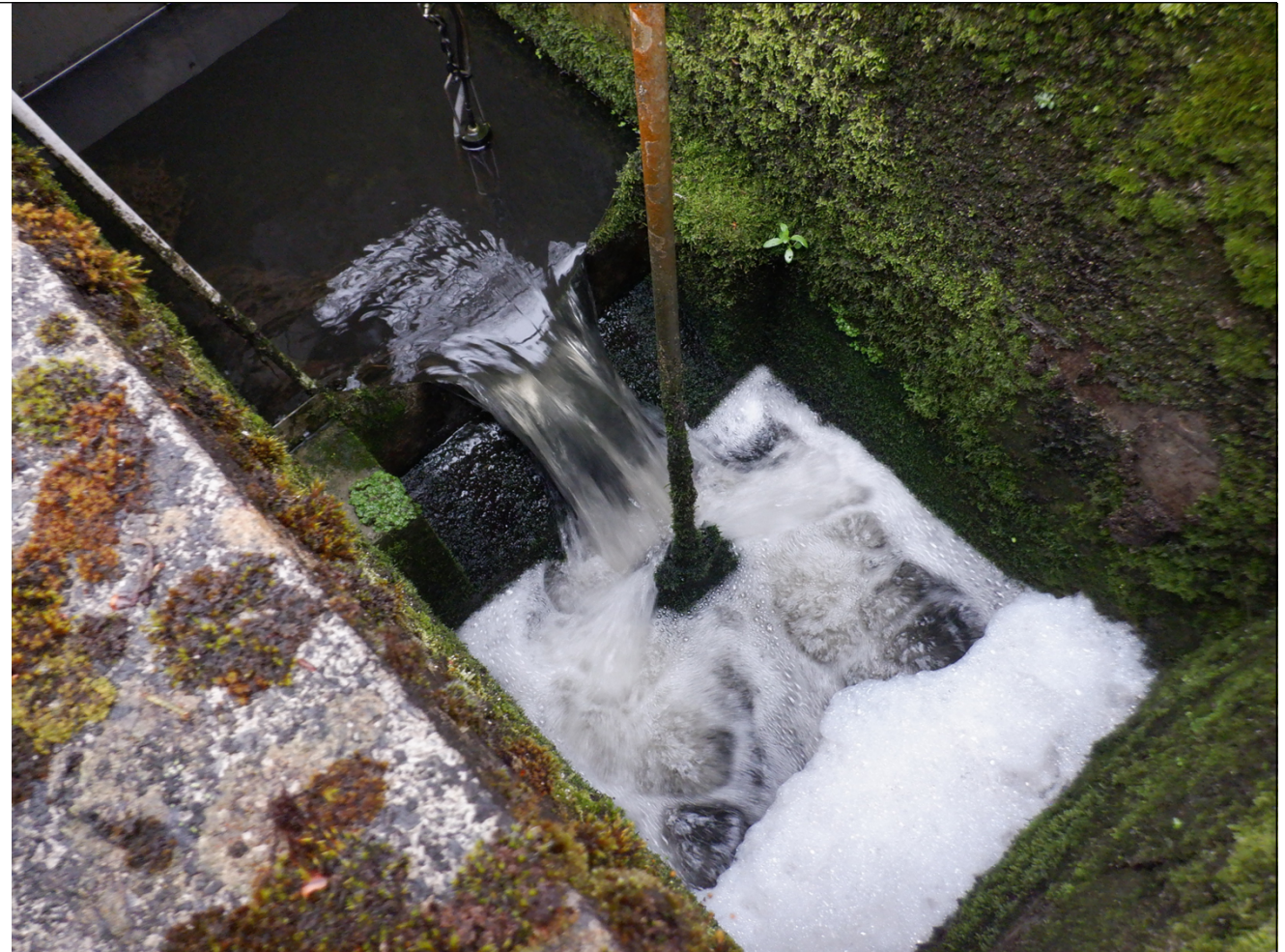
Figure 7 Final effluent sampling point.
