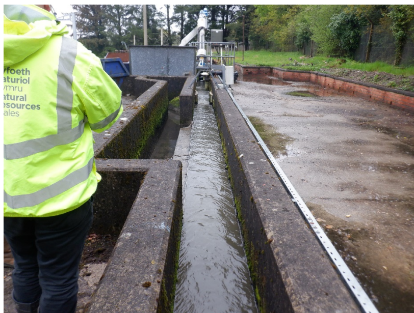
Figure 1: Inlet to the works with CSO overflow weir on the left.
