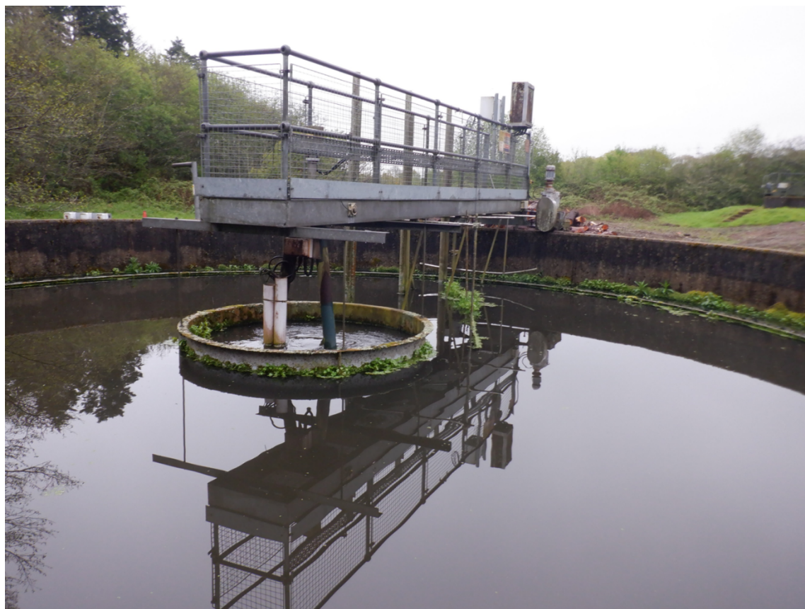
Figure 6 Final effluent tank
