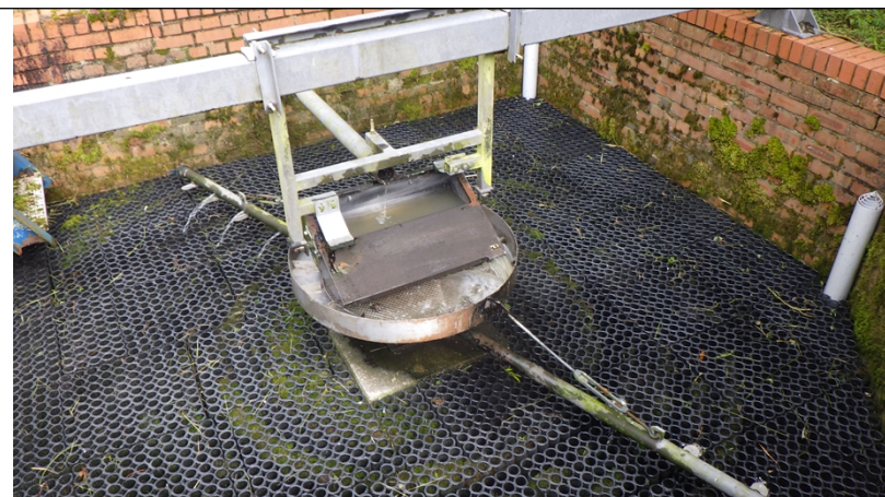
Figure 1 – Site visit photo: Filter arms working as designed.
