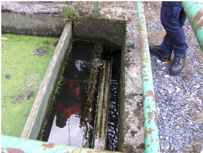
Image 4 – final settlement tank weir.
