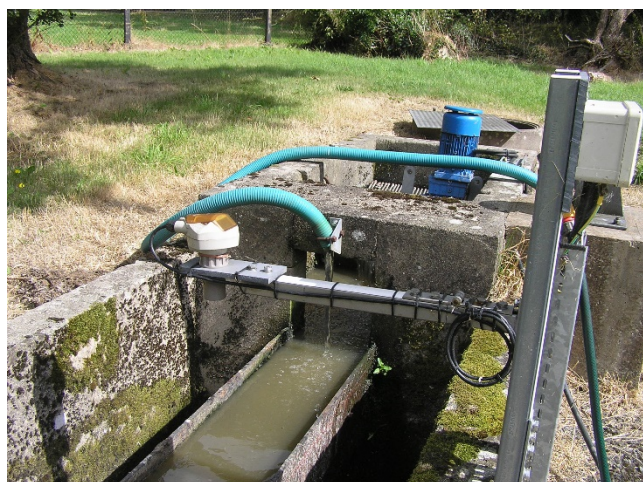
Image 1 – Inlet and re circ in operation
