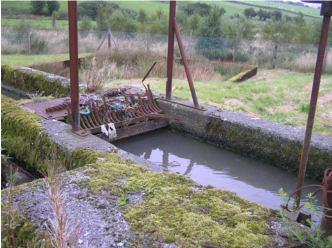
Image 1- Inlet screen in disrepair.
