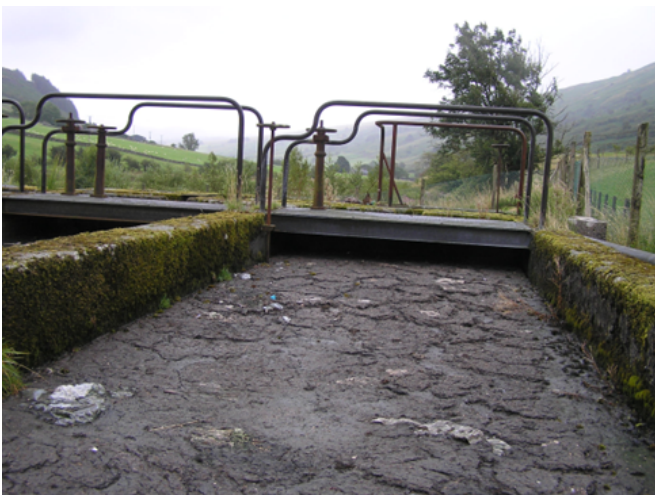
Image 2 – primary tanks with sanitary products
