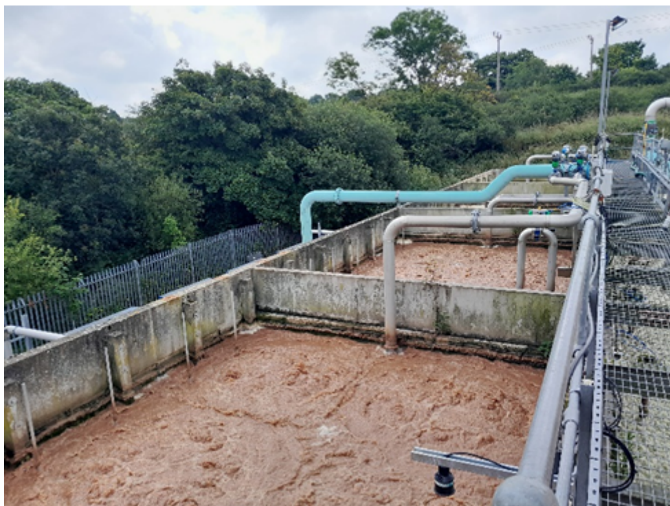
Image 08 – Recently commissioned MBR filters operational.
