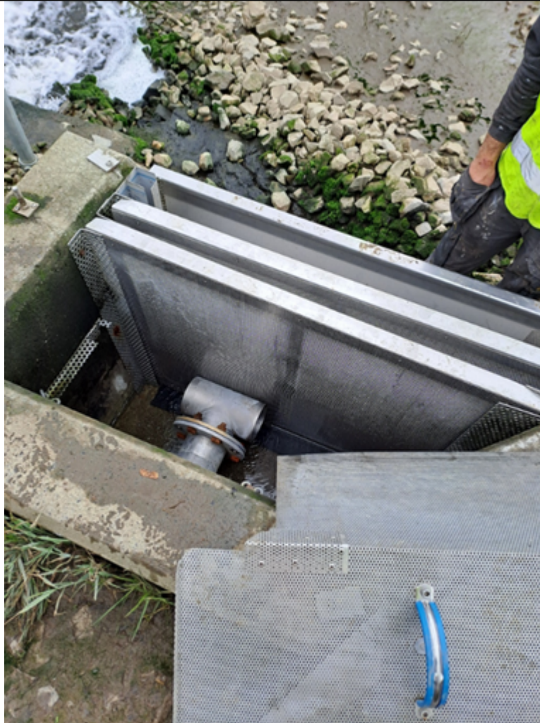
Image 01 – First Milk outfall with the screen removed in preparation for cleaning and inspection.
