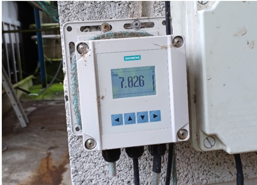
Image 5: Sludge Tank Level Sensor
