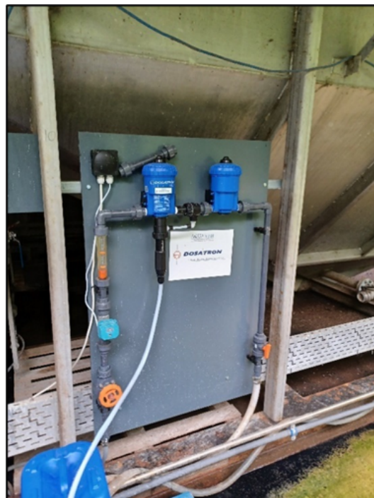
Image 4: ETP Dosing System
