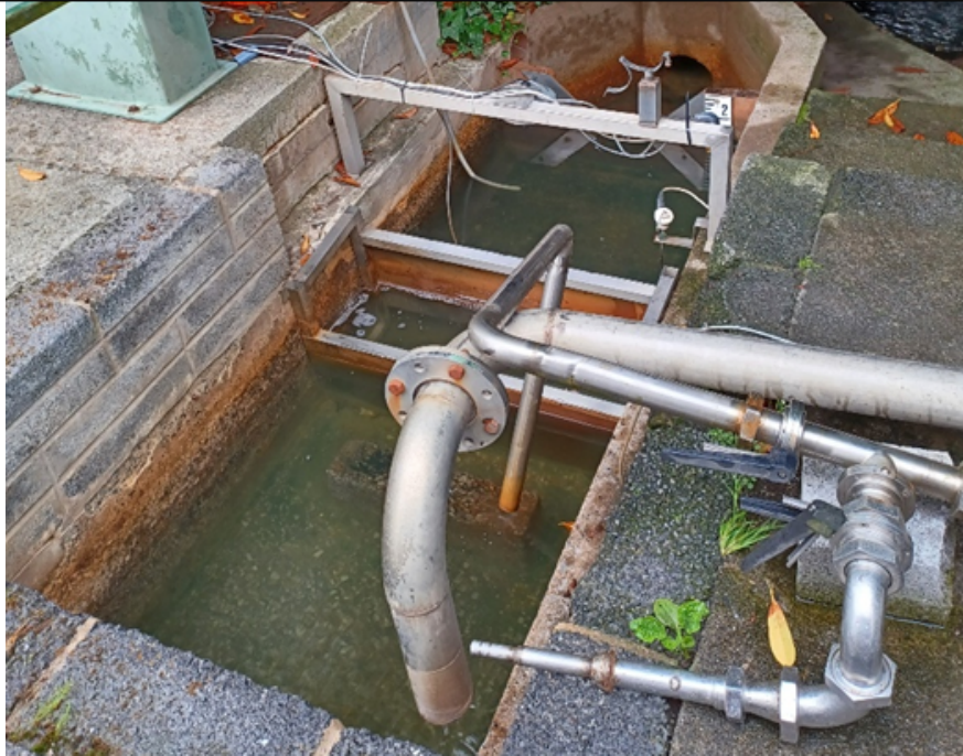
Image 6: V-Notch Flow Meter Chamber
