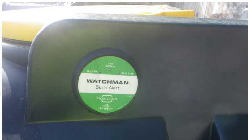
Photograph of warning device attached to oil container.
