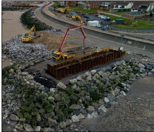
Figure 4 - Sheet piling cofferdam recently installed at East Rhyll using the similar installation methodology.
