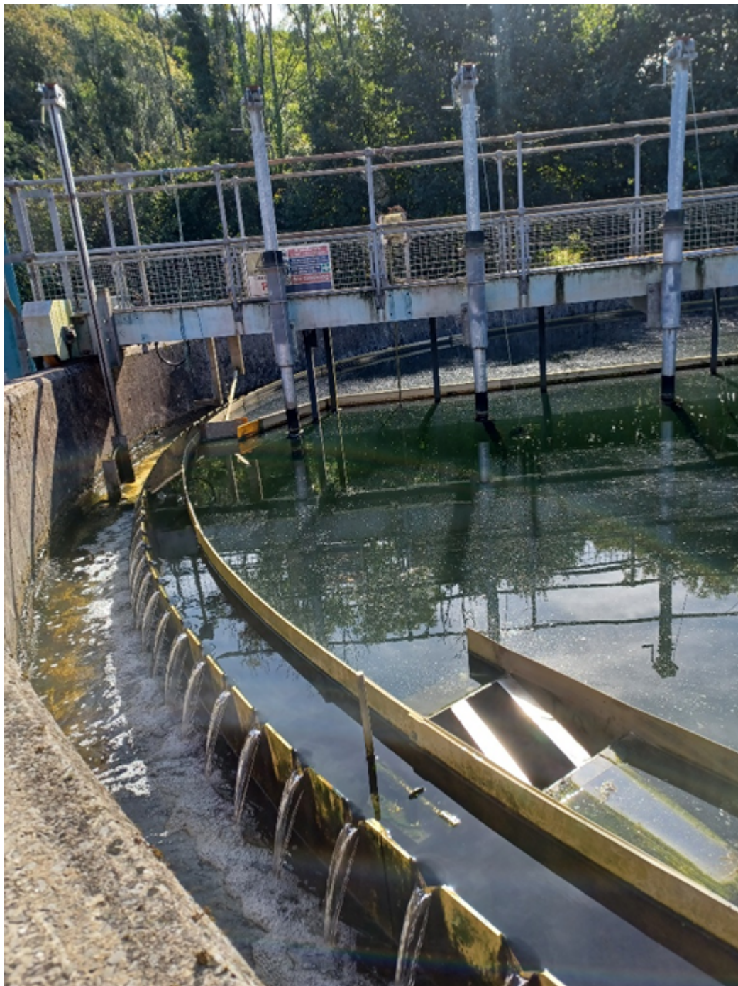
Figure 4 – Final settlement tank
