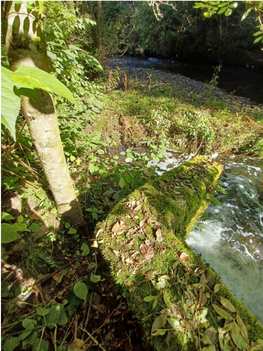
Figure 7 – erosion to the left of the headwall.
