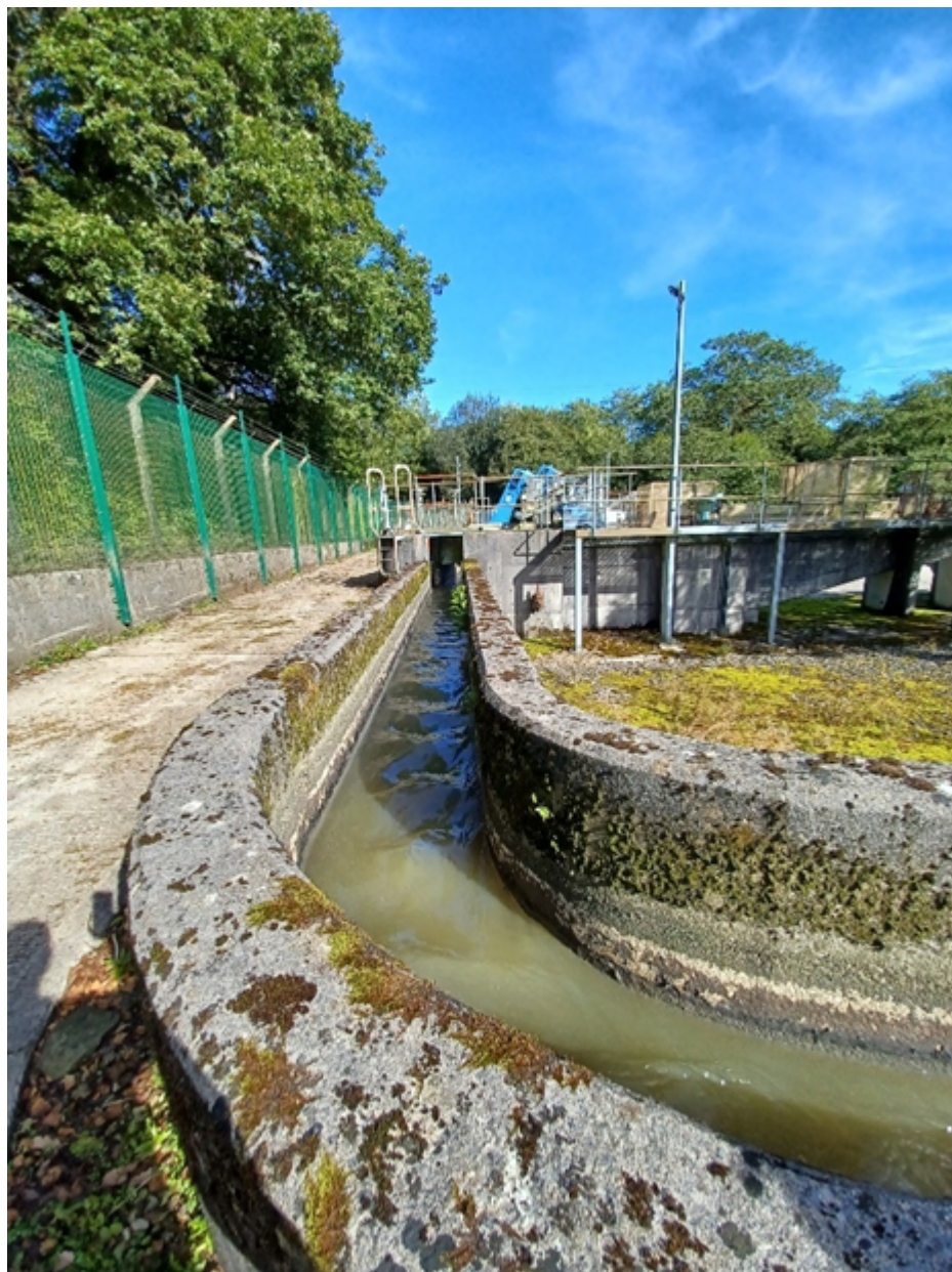
Figure 1 – wastewater after screens
