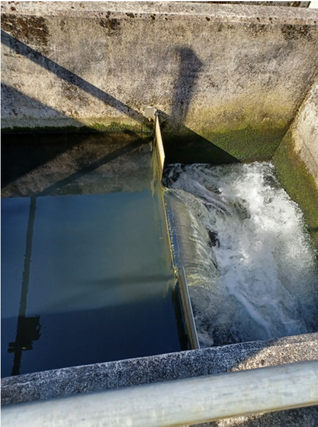
Figure 5 – final effluent prior to outfall
