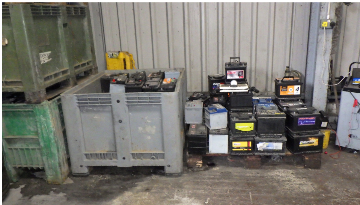
Batteries stored indoors.
