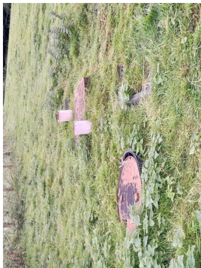
Septic tank location (Fig 1)
