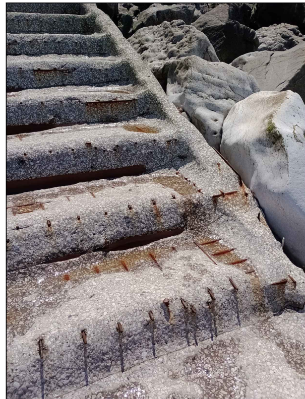
PHOTO 3 - VIEW OF EXPOSED REBAR ON RIGHT OF STAIRCASE
